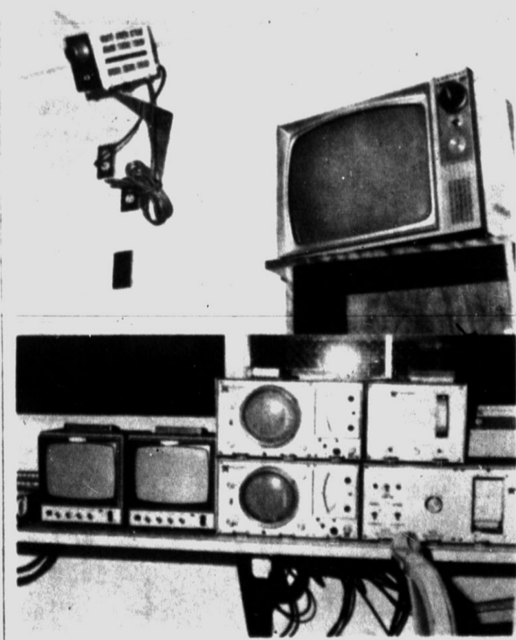
CLOSED CIRCUIT TELEVISION — Deaf Smith County Hospital has included two units which will visually monitor heart patients at all times, in conjunction with their recently installed coronary care equipment. At top left is the t.v. camera (alongside the patient's regular t.v. set) which transmits a picture onto the screens of the small sets at bottom left, showing the movements of the patients while lying in his bed. Administrator T. E. Seigler pointed this system out as offering far greater care to all heart patients.
