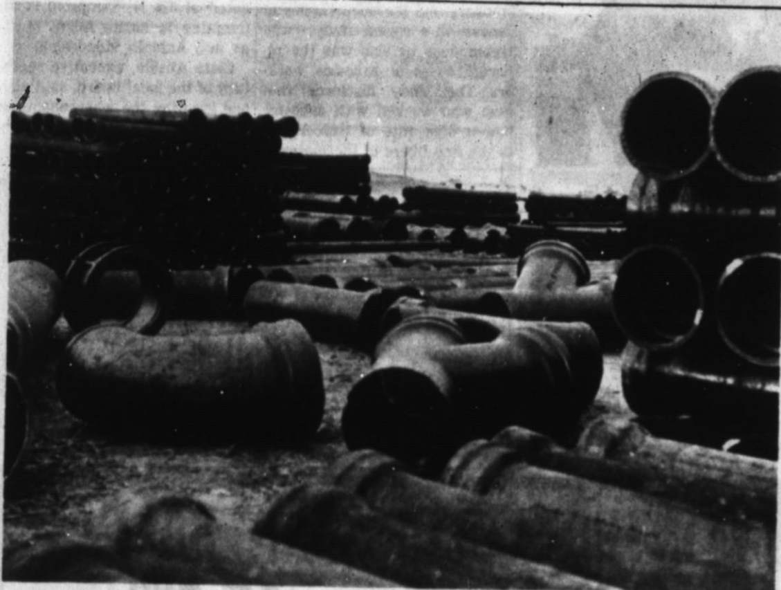
WILSON PLUMBING — This mass of confusion really isn't that mixed up, since workers at the Wilson & Co. construction site know exactly where each of these items will go. The plumbing facilities arrived last week and were stacked according to use and where they will go. —Staff Photo
