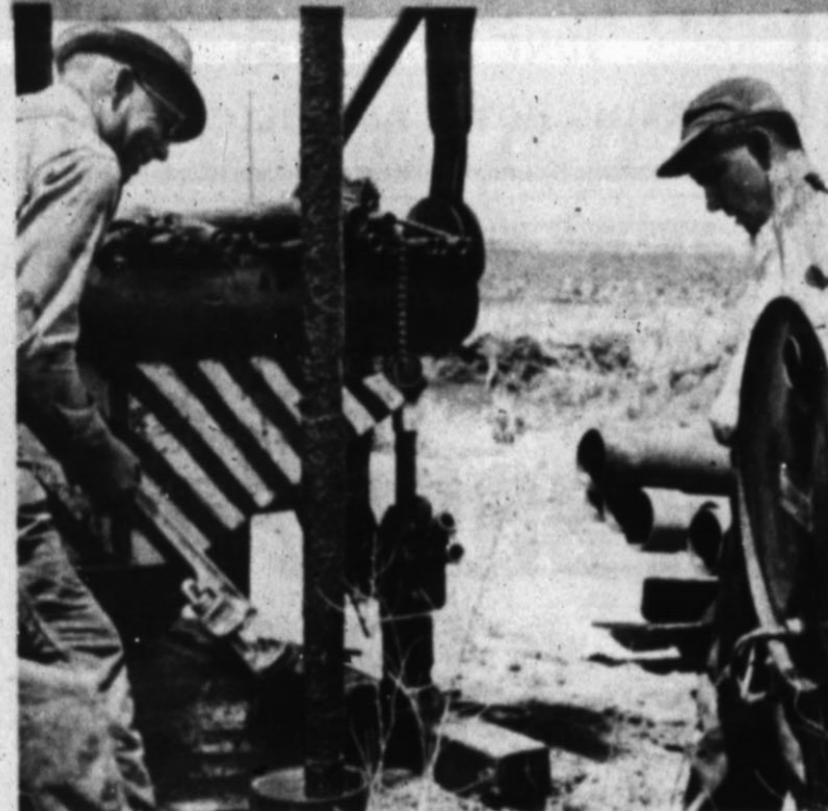
ONE OF THE most frequent aspects of Walco Drilling is cleaning or repairing a pump. Here, Jack Gray, left, and Lionel DeLeon, labor under a hot sun Monday pulling a pump out, west of Hereford. (Hereford Brand Photo)
