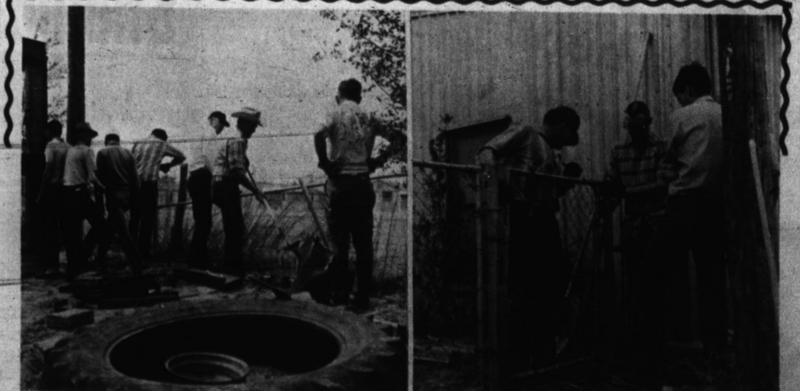
ASSIST TO THE MIGRANT MINISTRY — Members of the Melody Sunday School Class of the First Methodist Church of Hereford took time off Saturday to move and erect a new fence at the Casa De Amigos. An addition is being added to the Migrant Ministry's building and the fence had
