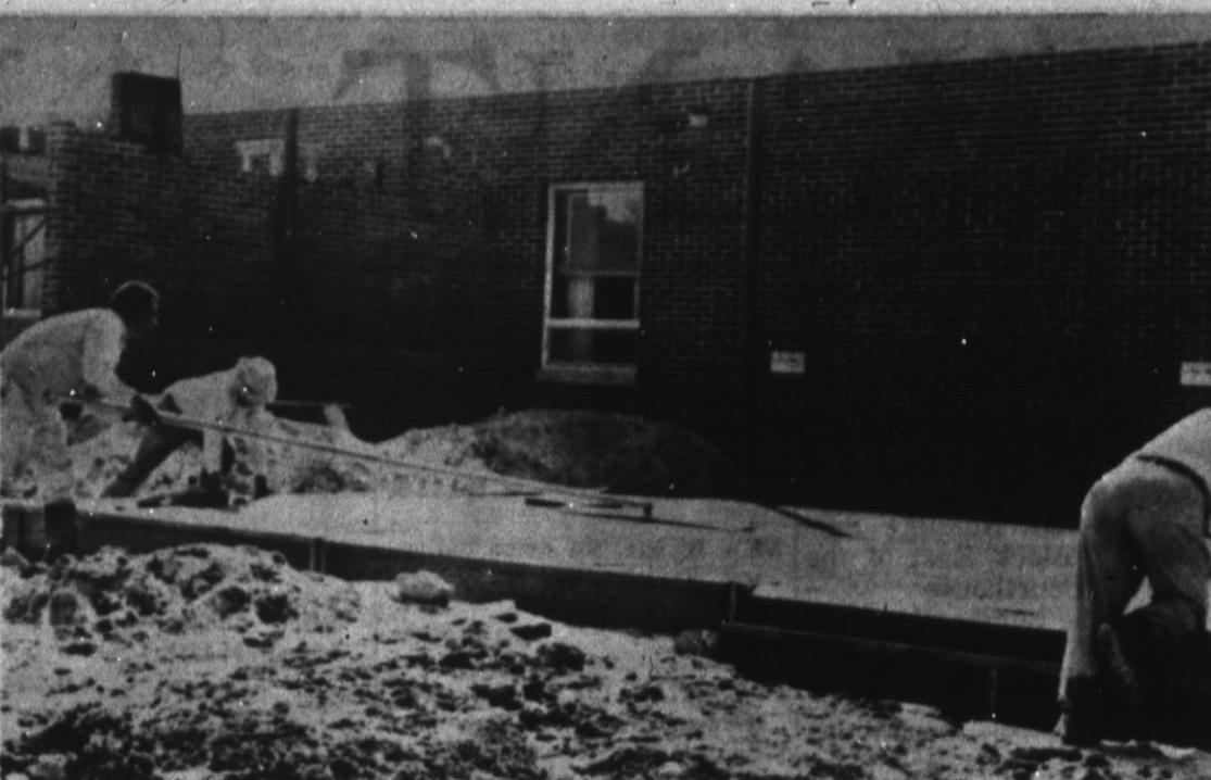
HOSPITAL PROGRESS — Workmen are shown here leveling the new concrete floor for the addition to the rear of the Deaf Smith County Hospital. Some of the walls have already begun to mark off the new space.
