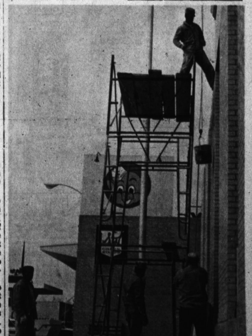
PROGRESS REPORT — Stone coping and plastering operations this week moved new construction on Post Office enlargement into finishing phases. (Hereford Brand Photo)
