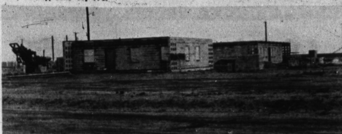
CAMP AT DIMMITT — A $1-million dollar complex gets above the ground as work progresses on the labor housing project. (Hereford Brand Photo)
