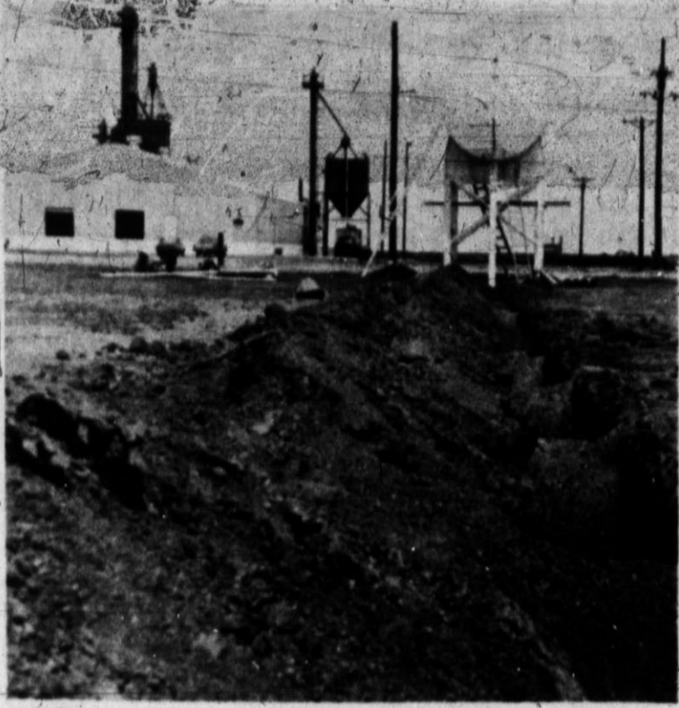
—Hereford Brand Photo SIGN OF PROGRESS — Construction at the location of new facilities for Pacific Molasses Co. was expected to have been completed Saturday and ready for operation this week. The thru-put plant includes the 25,000 gallon tank in the picture and two similar ones underground.
