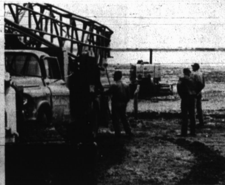
EQUIPMENT UNDERWATER — Employees of the Messer Construction Co. worked Friday morning pulling digging equipment from high waters on the Luther Lesly farm about 1 1/2 miles east of Milo Center. A bulldozer is being pulled from the water.
