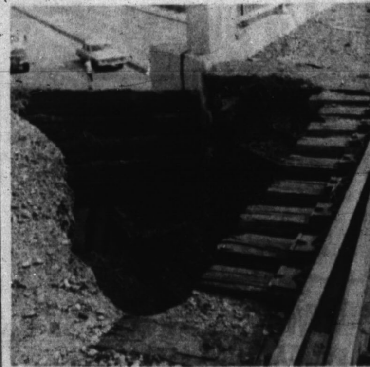
RAIN PROBLEMS — Hereford residents had their problems as the result of heavy rains late Thursday night and early Friday morning. Scenes show, at left, a washout of the
