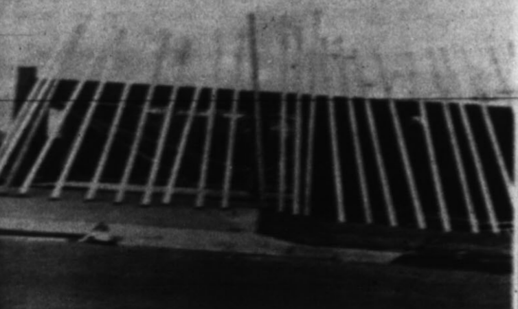
Home going up in 100 block of Juniper Street . . . Westhaven Addition—more Hereford on the grown.
