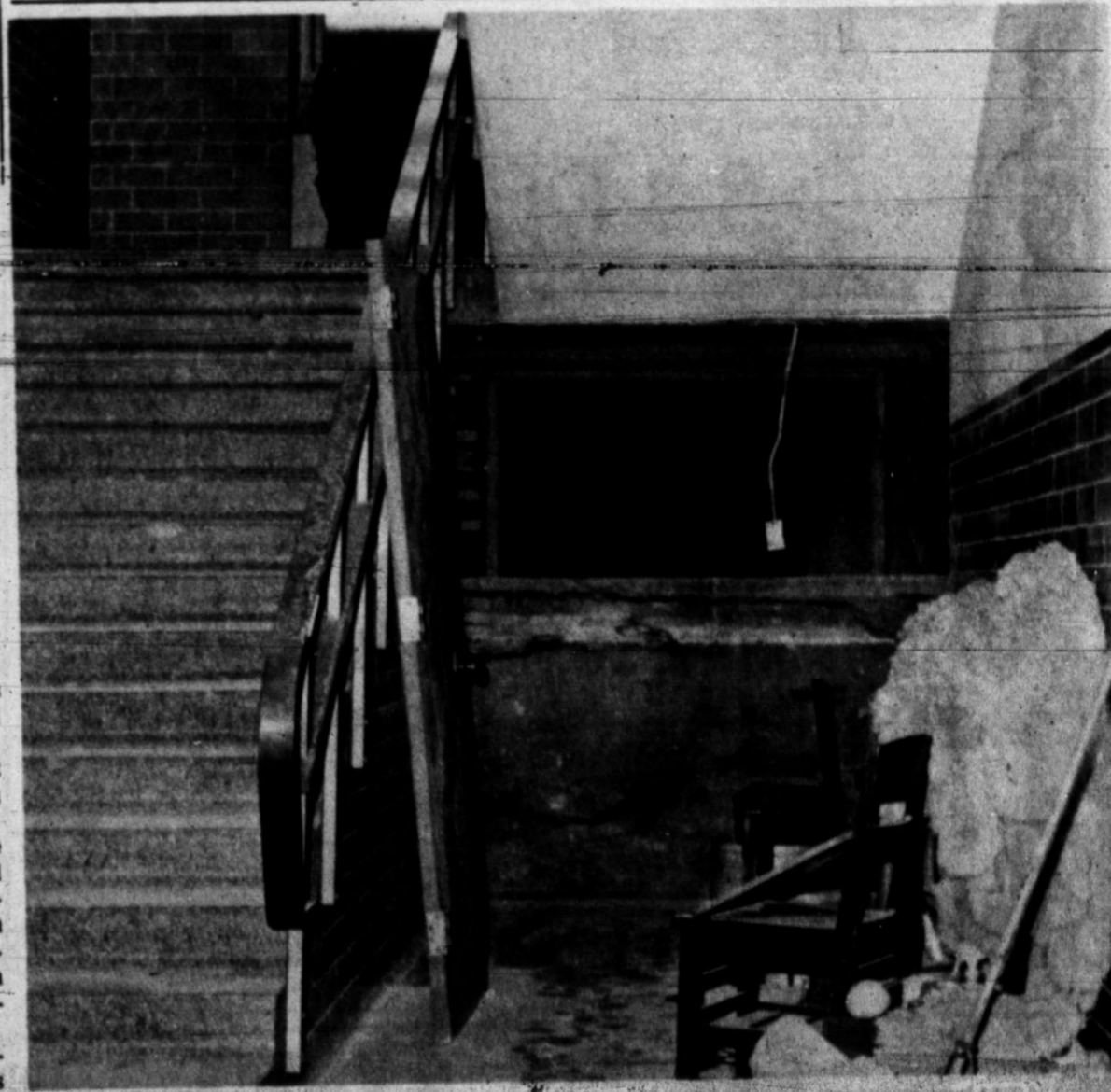
BUILDINGS TOGETHER — Addition of the vocational building will join all high school facilities on the academic campus under one roof. Here an entranceway has been cut to join corridors between the new and existing buildings.
