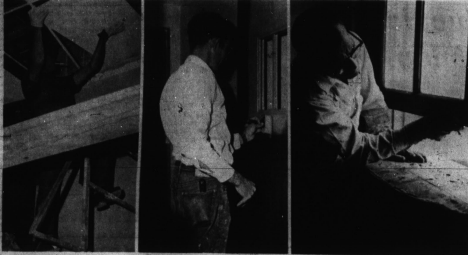
SIGNS OF PROGRESS — Workers at the post office building continue work at a fast pace in order to finish the remodeling by the early part of June. Many pieces of new
