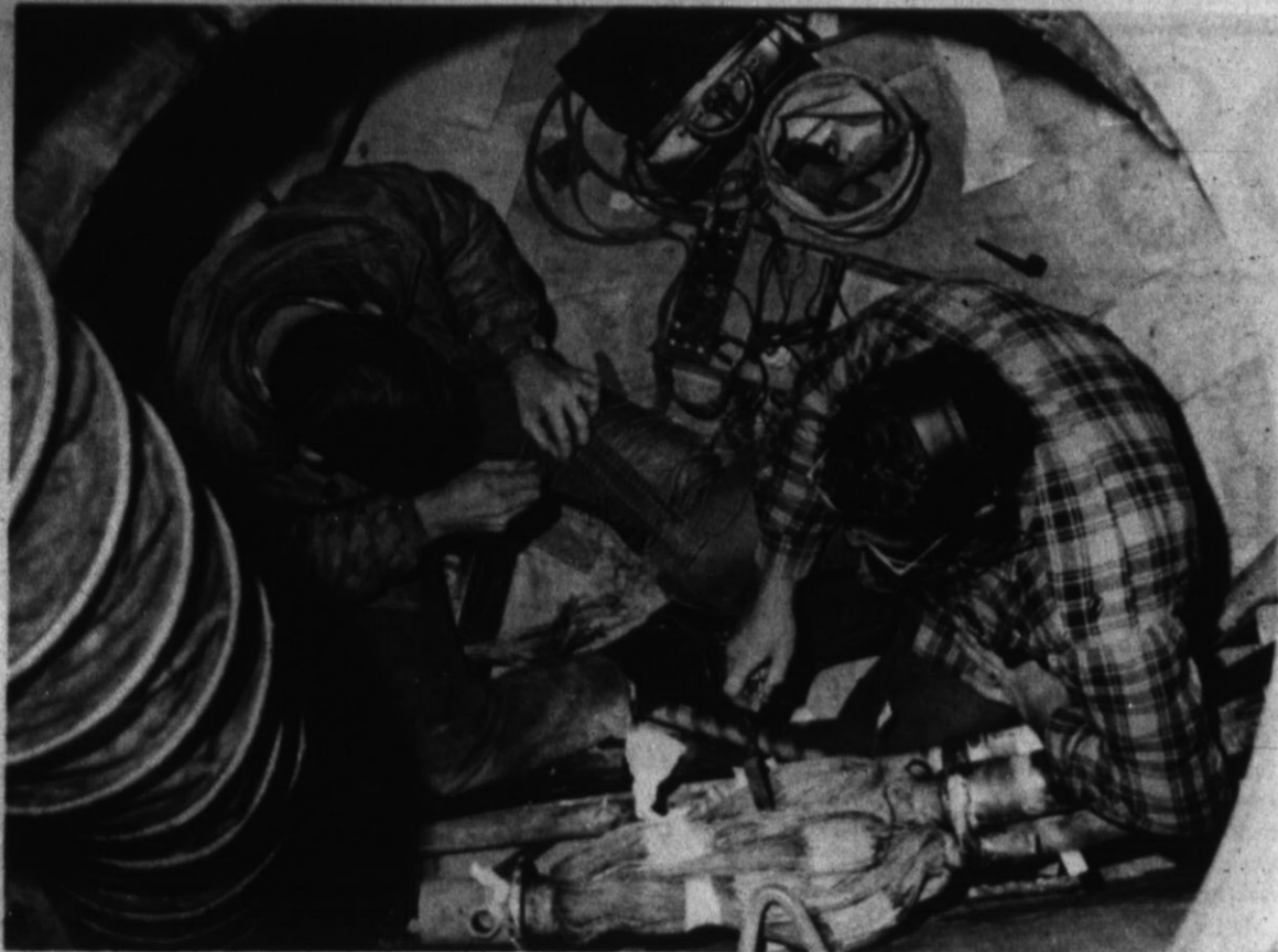
CABLE SPICERS — These two men, called cable spicers because of the work they do, were in Hereford and in a manhole during the last few weeks. The two are from Amarillo and were adding a 600 pair cable to one of the main lines of the telephone company. Work such as this is done depending upon how rapid the town or a certain section grows. (Hereford Brand Photo)
