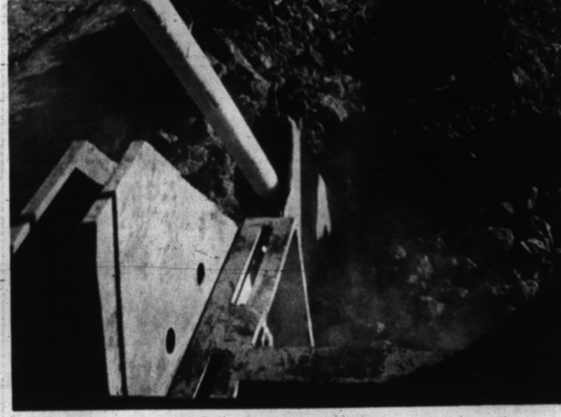
ONE OPERATION — Plastic pipe line is laid in one operation with this hollow blade made by Bryant Brothers Pipe Line Construction. Dean, Kenneth and Tommy
