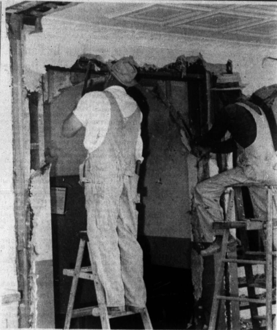
REMODELING BEGINS — City employs the first floor of Hereford City Hall. (Staff and carpenters begin the renovation of Photo)
