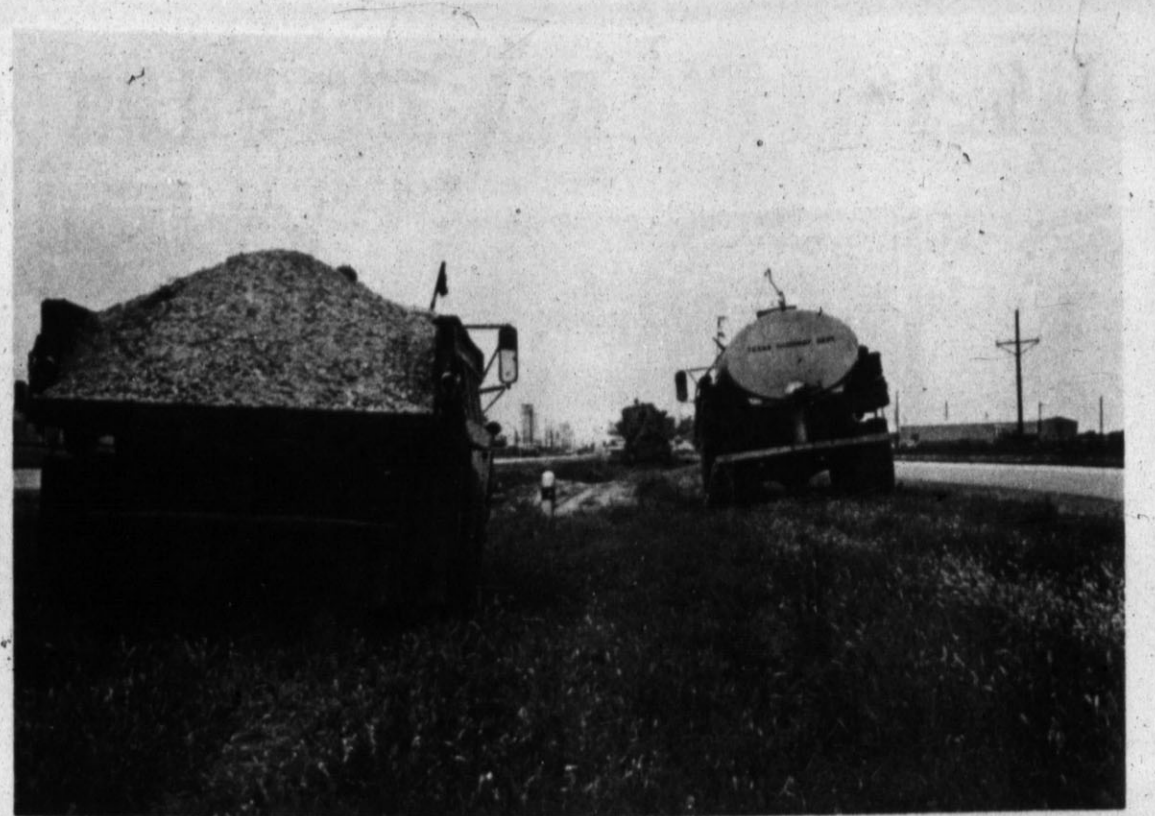
SIGN OF PROGRESS — Extra median crossings are being added to U.S. 60 just east of the city this week by the Texas Highway Department. A highway engineer said the extra additions would give a uniform number of median crossings from the city limits to the Hereford Feed Yards. (Hereford Brand Photo)
