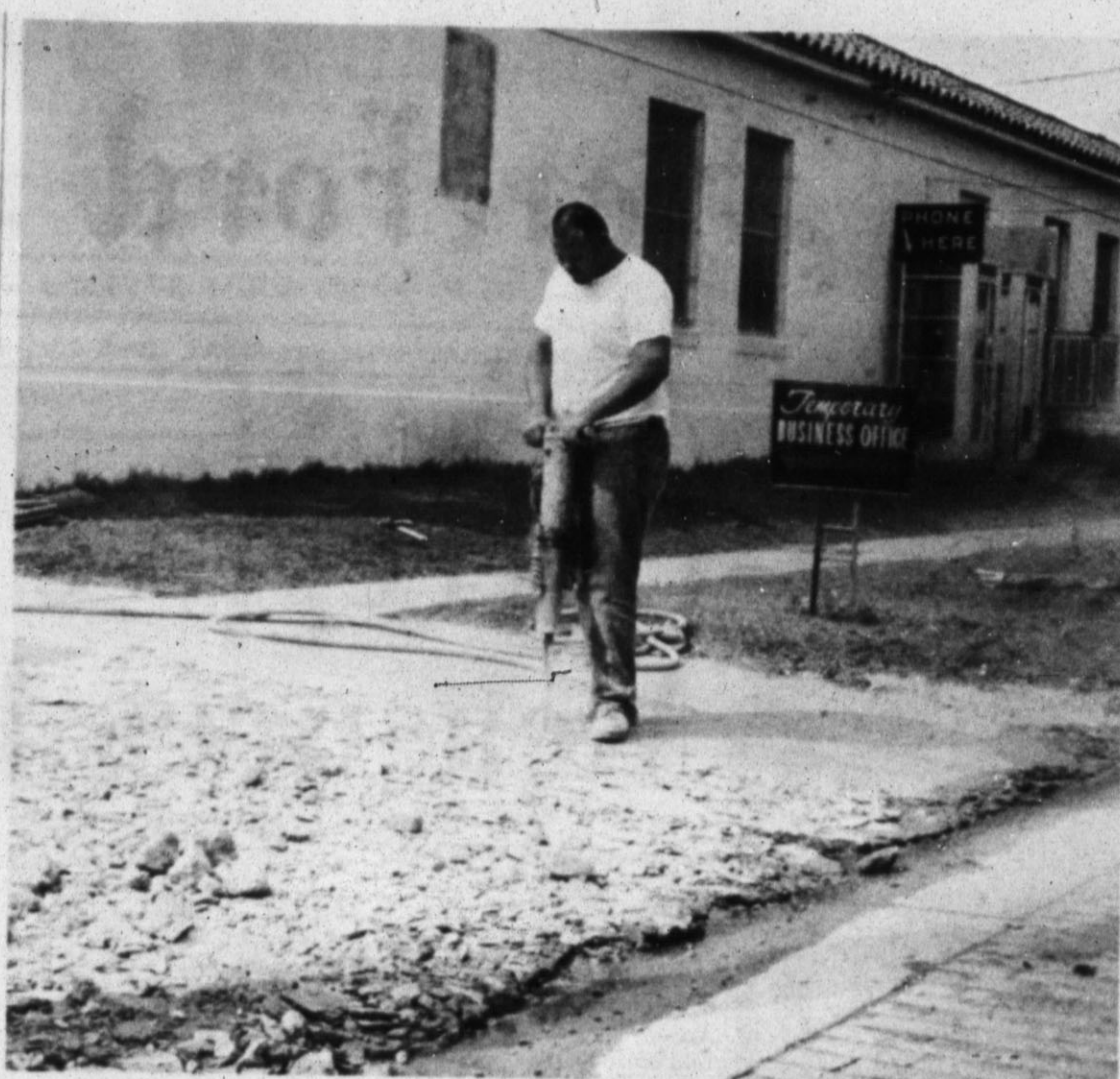
SIGNS OF PROGRESS — Part of many construction jobs requires tearing out of one part to make way for a new addition. The steady tattoo of an air-hammer reverberated through downtown Hereford early this week as workers removed part of the sidewalk north of Southwestern Bell Telephone. The addition is a double drive to a service area. (Staff Photo)
