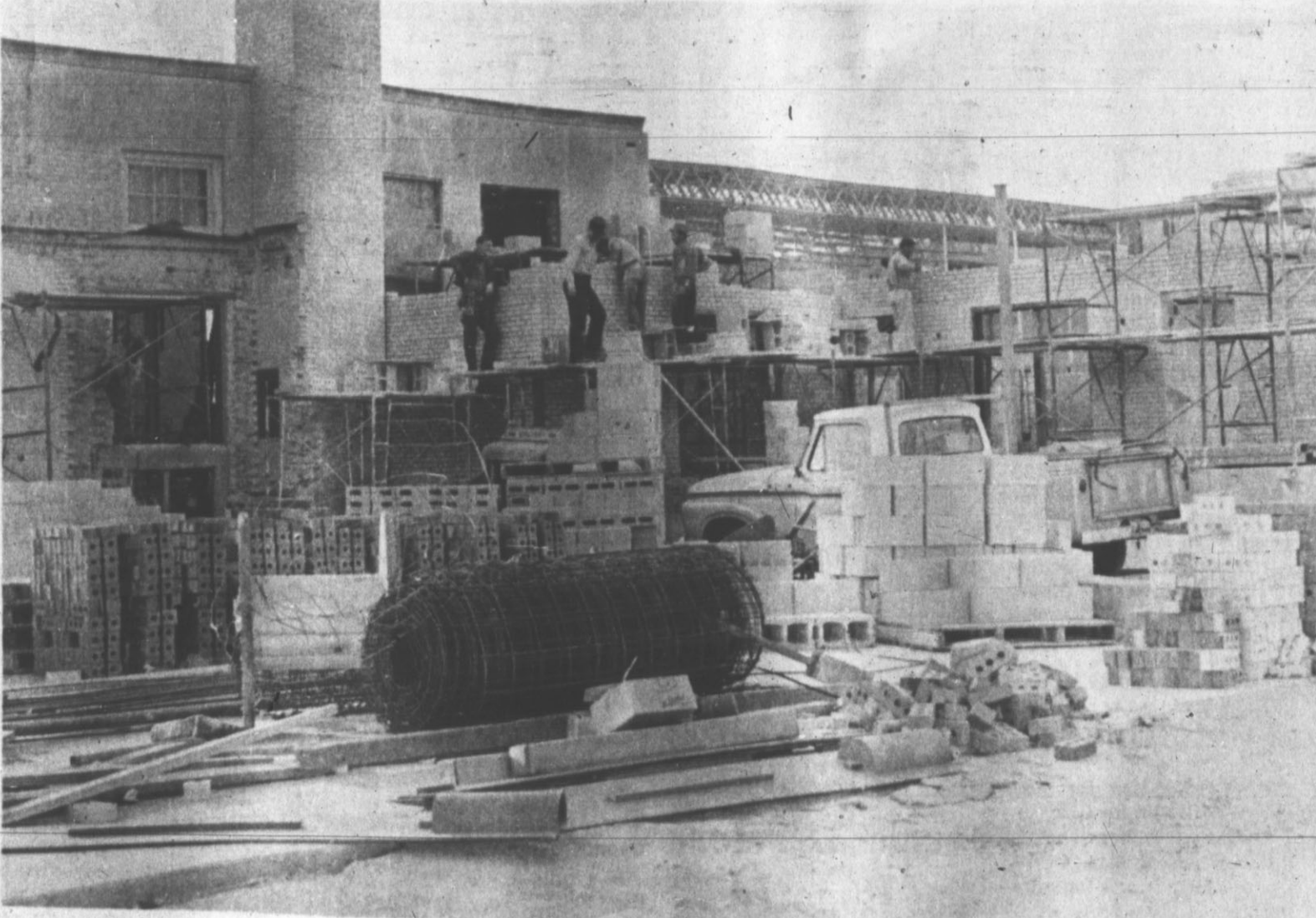
PROGRESS REPORT — Walls of the Post Office addition are pushing up in what appears to be mass confusion, but workers keep it sorted out and each seems to be accomplishing what he sets out to do. The structure is following design established by the old building, and even some of the older windows are being used according to a post office employee. (Hereford Brand Photo)
