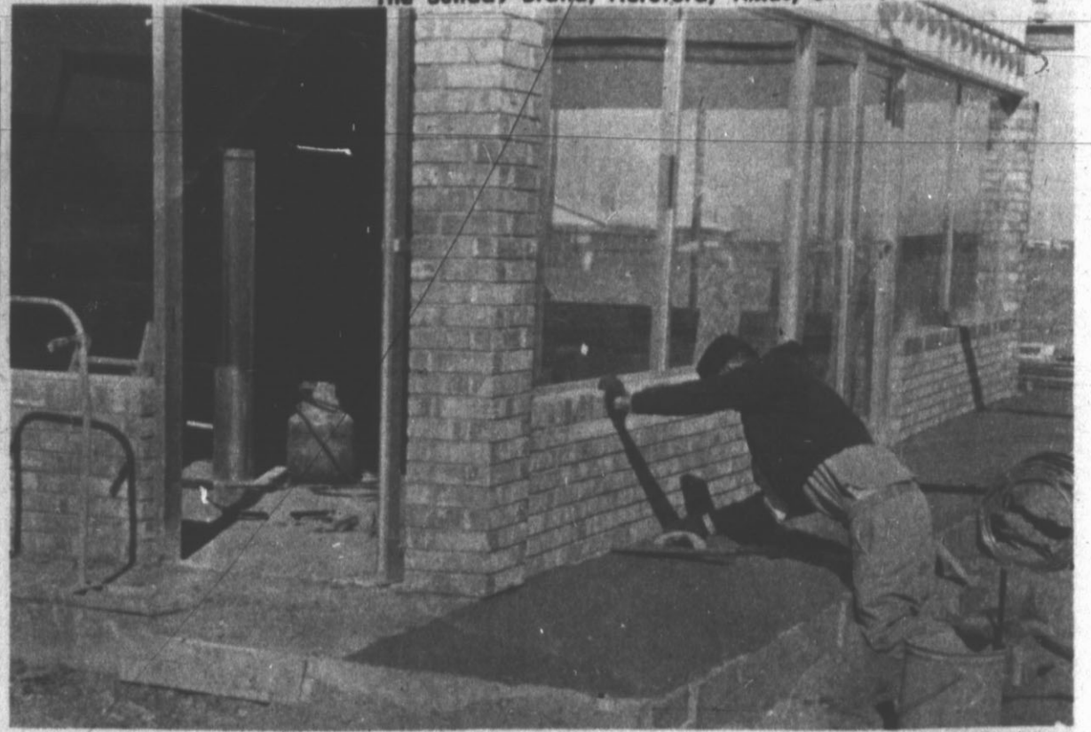
SIGNS OF PROGRESS — A new drive is being built on north 385. J. W. Robinson and Bill Gentry are partners in the project which is being built by Kruse-Reed Construction Co., of Plainview. This is the same firm that built Robo, the car wash that is located just south of the new drive in cafe. (Hereford Brand Photo)
