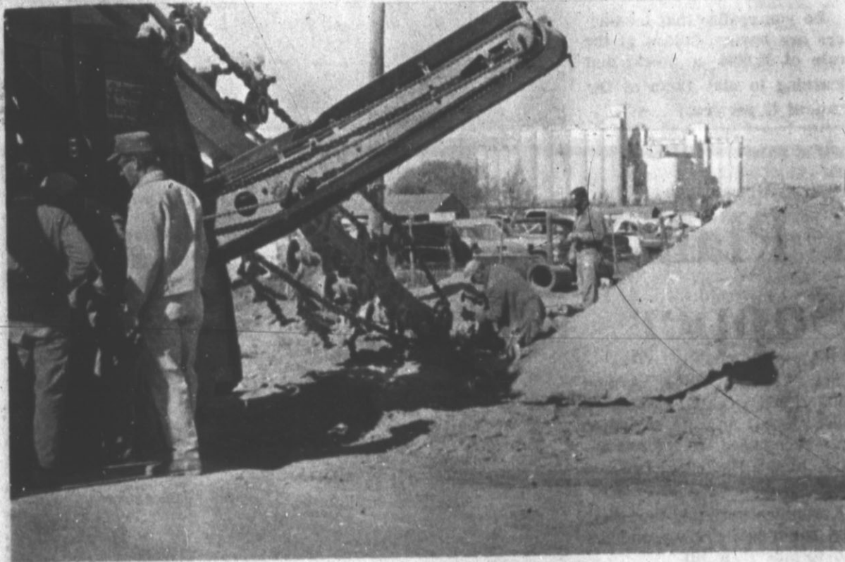
EXTENDED CITY SERVICE — Municipal water and sewer service is being extended to south Hereford, across Tierra Blanca Creek. Shown is equipment belonging to H. B. Jordan, Inc. of Amarillo, low bidder for the sewer and water construction. The sewer and water phase of the program was let for $517,807.67. The project was advanced south to Austin road at the end of this week. (Hereford Brand Photo).
