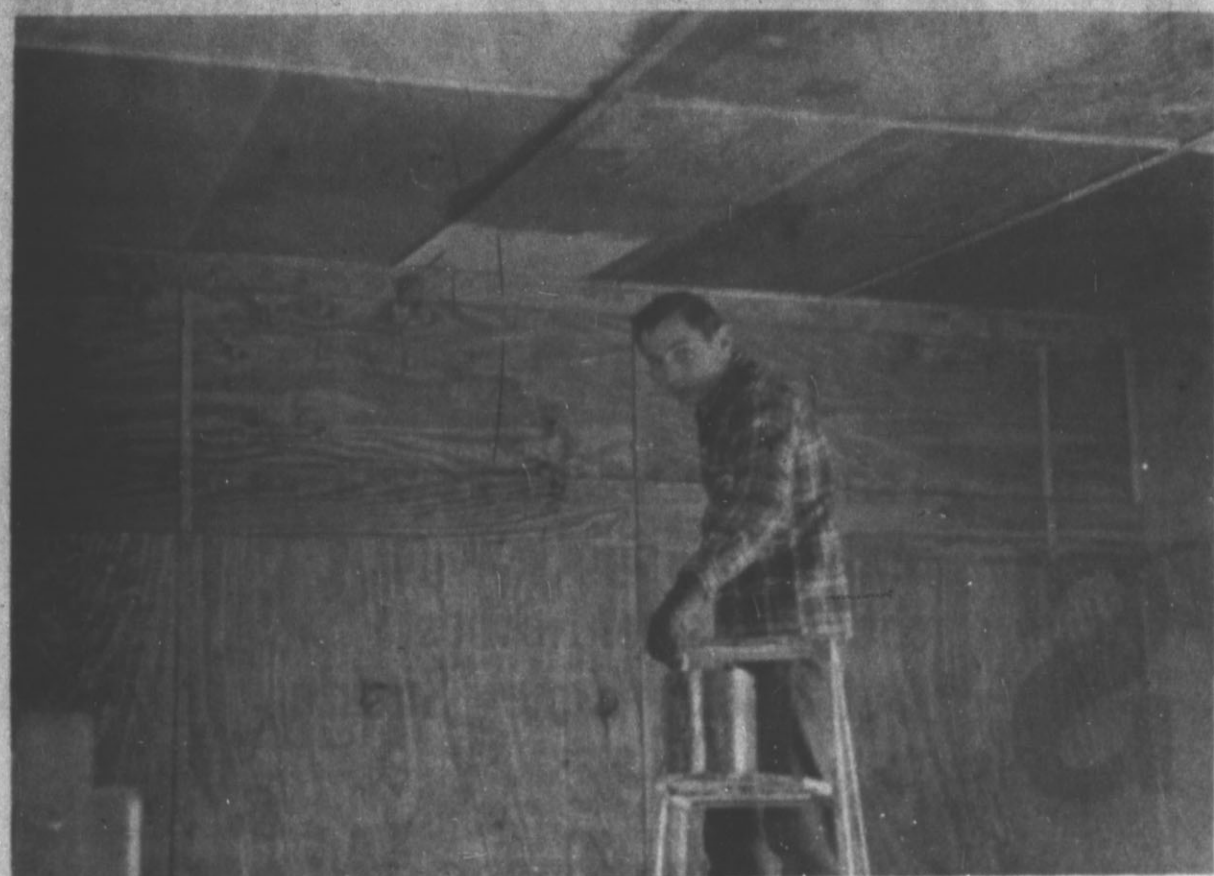
REBUILDING — Hereford Fruit Market, damaged extensively by fire earlier this fall, is building a new building behind the original structure. Floor space has been almost doubled and has modern, stained paneling interior. The bottom photo shows Darrell Martin staining the panels over the meat market area of the building. (Hereford Brand Photo)
