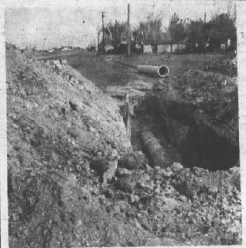
WATER LINES GOING DOWN — Water lines began going down during the past week as the city has begun to tie in the newly developed northwest part of Hereford with the large booster station. Final connection on the lines should be made by January, said City Manager Dudley Bayne. The construction area pictured is on Plains Avenue looking east. (Hereford Brand Photo)
