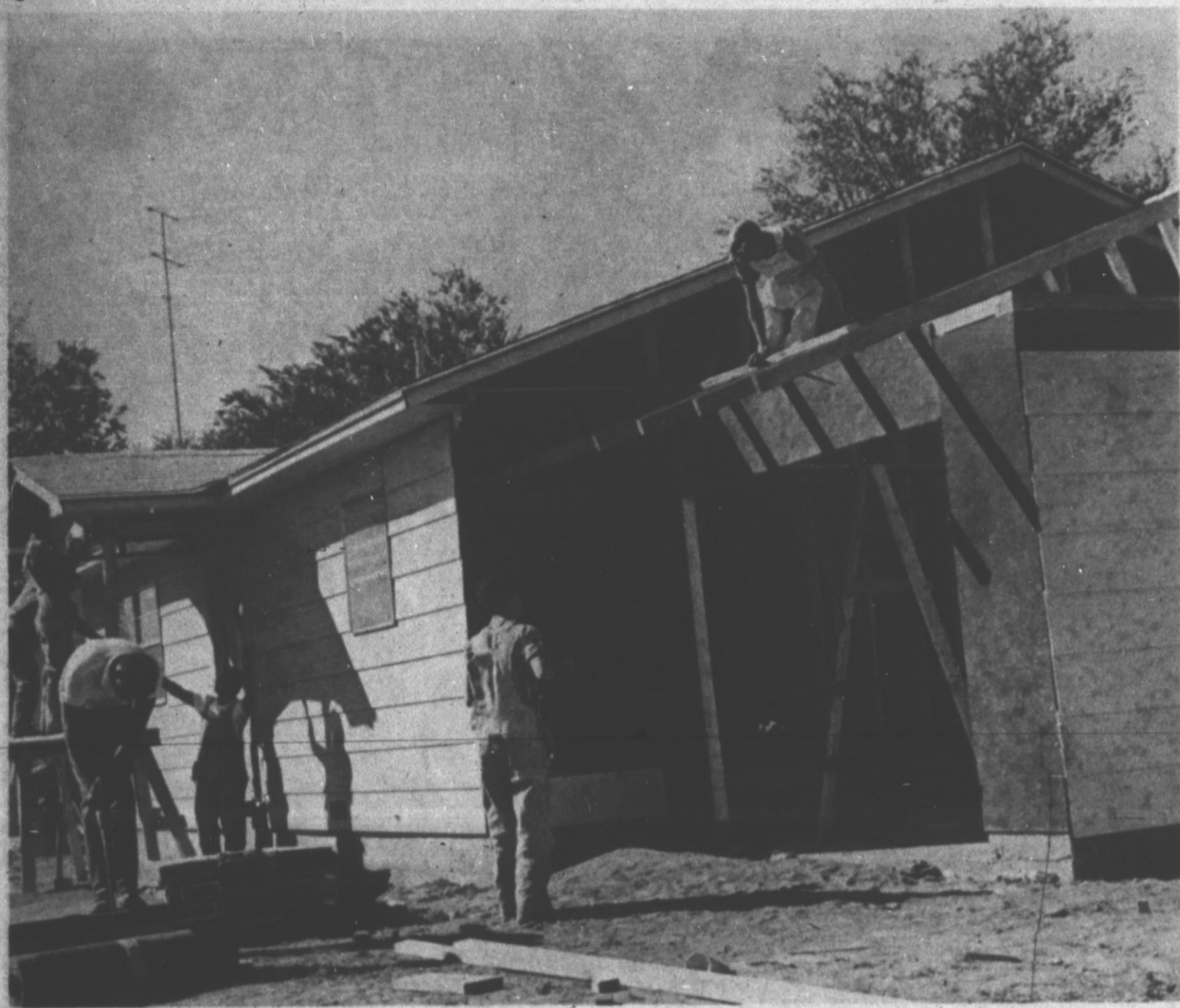
PROGRESS REPORT — These high school boys working in the new vocational program are going right up with their house. The house being constructed during class time is
