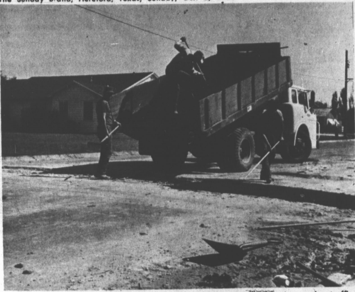
SIGN OF PROGRESS — City employees were doing "patchwork" this week between Ave. J and Star Street as a waterpipe excavation was being smoothed over for traffic. (Hereford Brand Photo)
