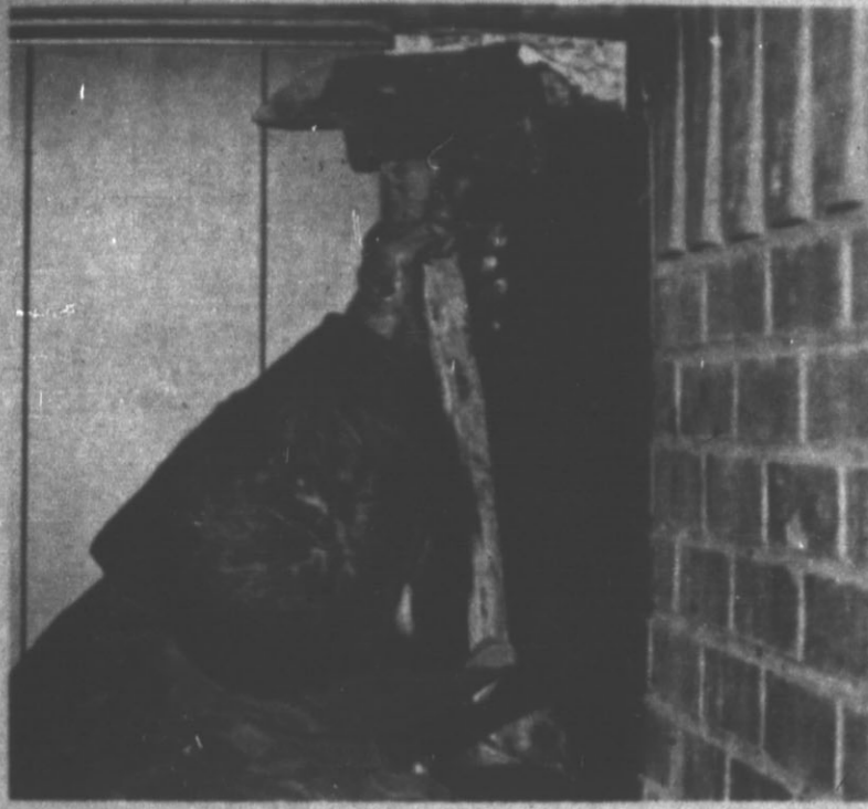
EXTENSIVE DAMAGE — A fire Saturday morning at the home of Bob Huddleston 114 Fir street, did extensive damage to the interior of the house. The Huddlestons were in Oklahoma at the time. The fire again erupted Saturday evening, sending the Hereford Fire Department back to the location a second time. (Hereford Brand Photo)
