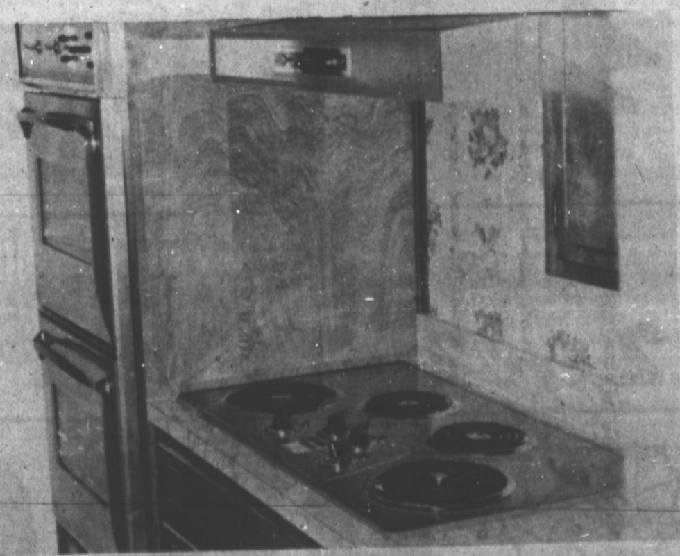
TOTAL ELECTRIC KITCHEN FEATURES BUILT-IN RANGE, DOUBLE OVEN, AUTOMATIC DISHWASHER, FOOD WASTE DISPOSER AND VENT HOOD.
