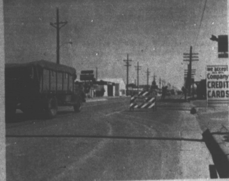
PATCHWORK BY HIGHWAY DEPARTMENT — The Texas Highway Department made good use of the dry weather in Hereford during the past week by painting new highway markers, building median crossings and doing general patchwork along U.S. 60 and 385. Workers were caught Thursday smoothing over rough spots in the 600 blocks along U.S. 60. (Hereford Brand Photo)
