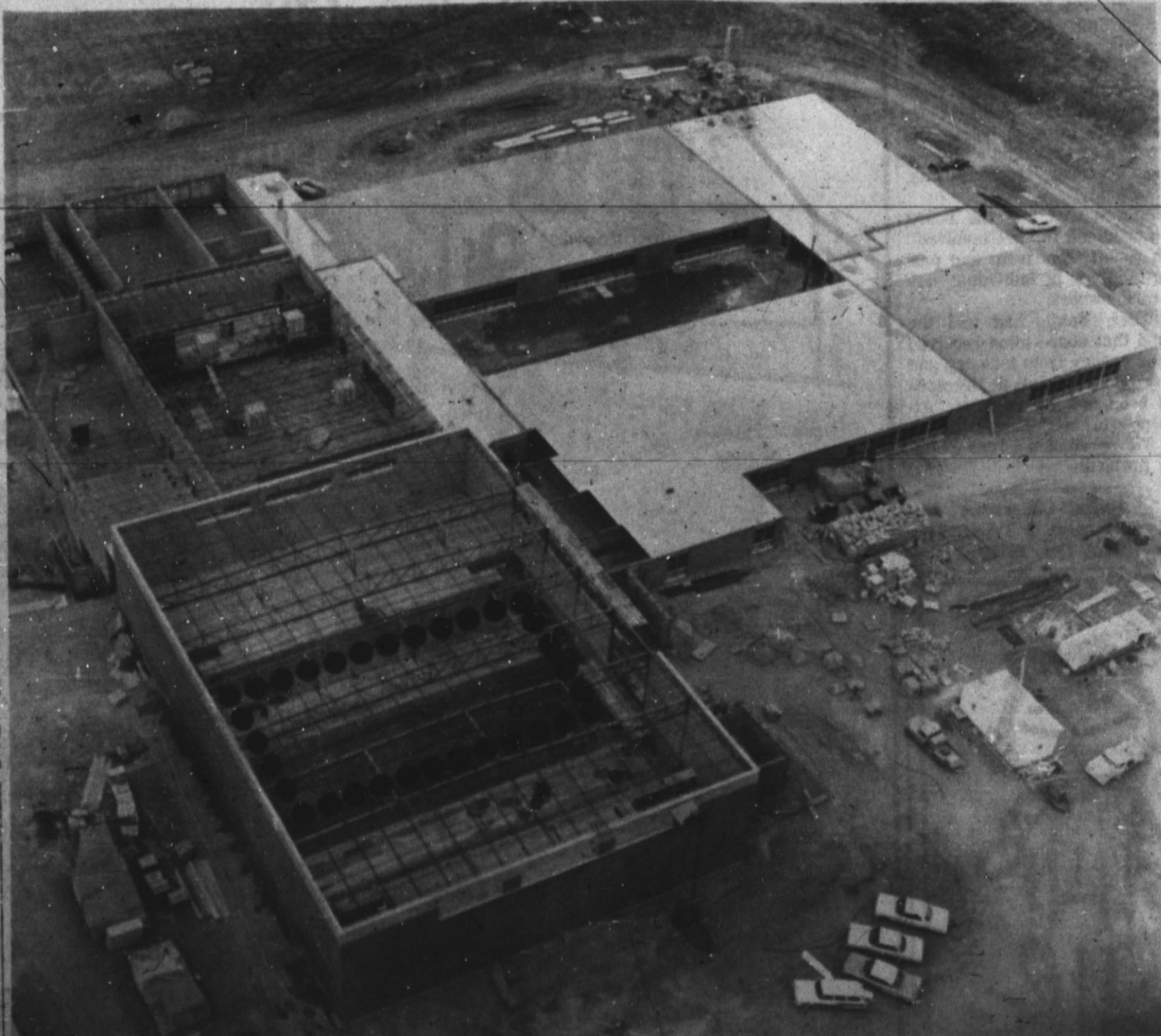
ROOM FOR 1800 — La Plata Junior High School, currently under construction in northwest Hereford, is rapidly taking shape, as this photo from the air shows. The large wing of the building at lower left is for the gymnasium, which will be home for Hereford High School basketball games following completion. The dotted line shows the approximate area of the basketball court. Remaining portion of the vast wing will house seating for some 1,800 persons or more. Dressing rooms will be constructed beneath the seating stands. The gym will also be home for the La Plata Junior High School Mavericks athletic teams. Completion is scheduled for July. (Staff Photo by Wain Miller)
