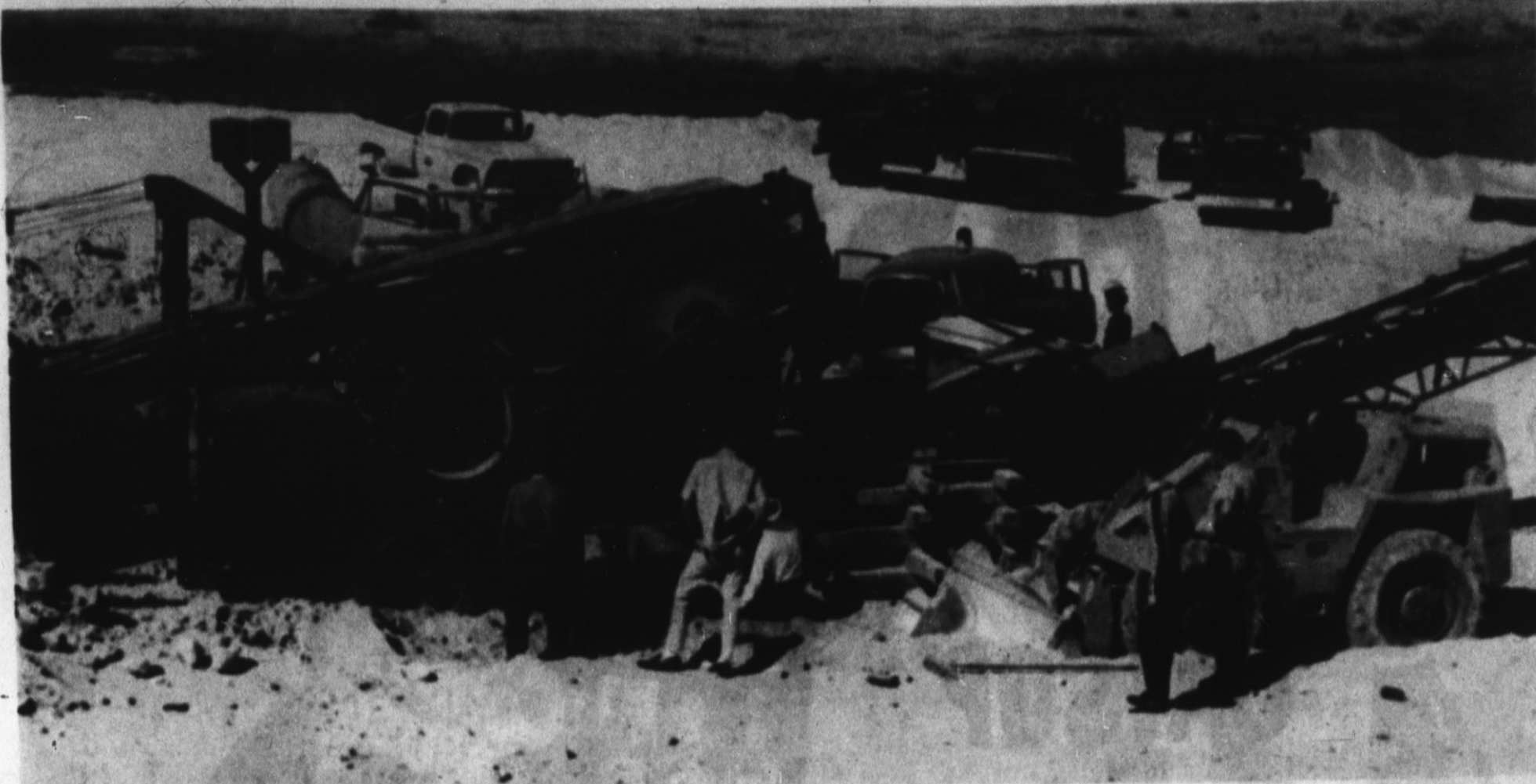
ACCIDENT SCENE —Rescue workers spent some 45 minutes working to free a man who became tangled in this large caliche-crushing machine near Hereford Monday. After being freed by rescuers working with cutting torches and jacks, Glen Polk, 24, was taken to Deaf Smith County Hospital for treatment of a seriously injured arm. (Staff Photo)
