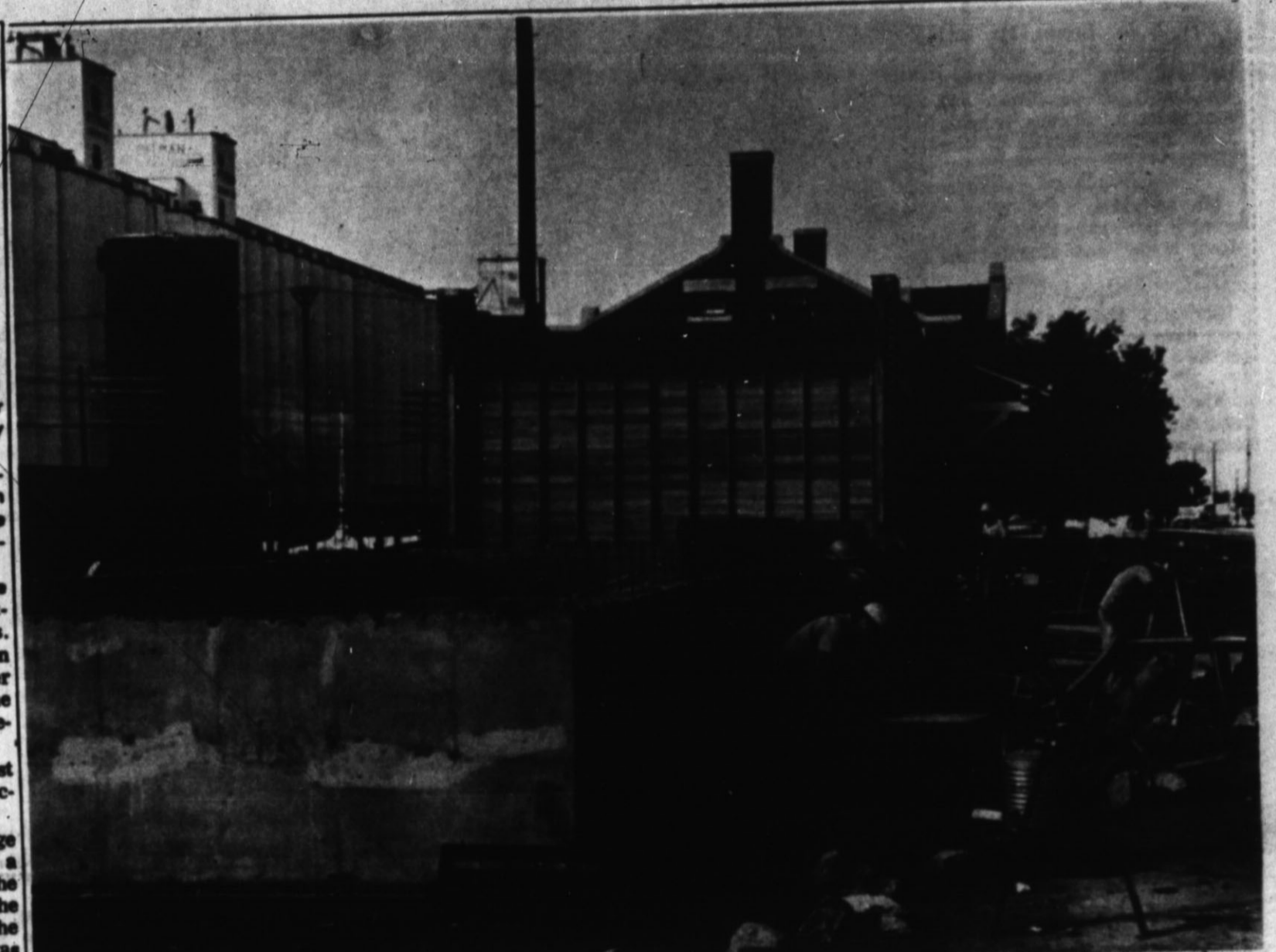
CONSTRUCTION BEGUN —Santa Fe construction workers began work on an addition to the Santa Fe Depot here recently and plan to finish the project in 60 to 90 days. The project not only includes this addition, which will be used for freight storage, but also the complete remodeling of the offices in the original part of the depot. (Staff Photo by David Butler)
