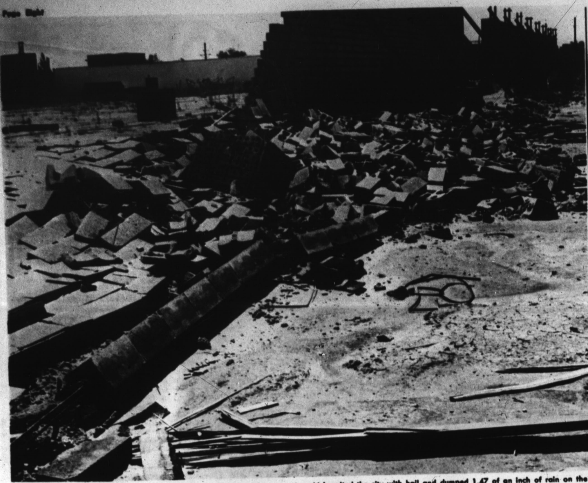
WIND DAMAGE —Two sections of concrete block walls at the Sugarland Mall Shopping Center were blown down in Sunday's windy thunderstorm which pelted the city with hail and dumped 1.47 of an inch of rain on the town. (Staff Photo)
