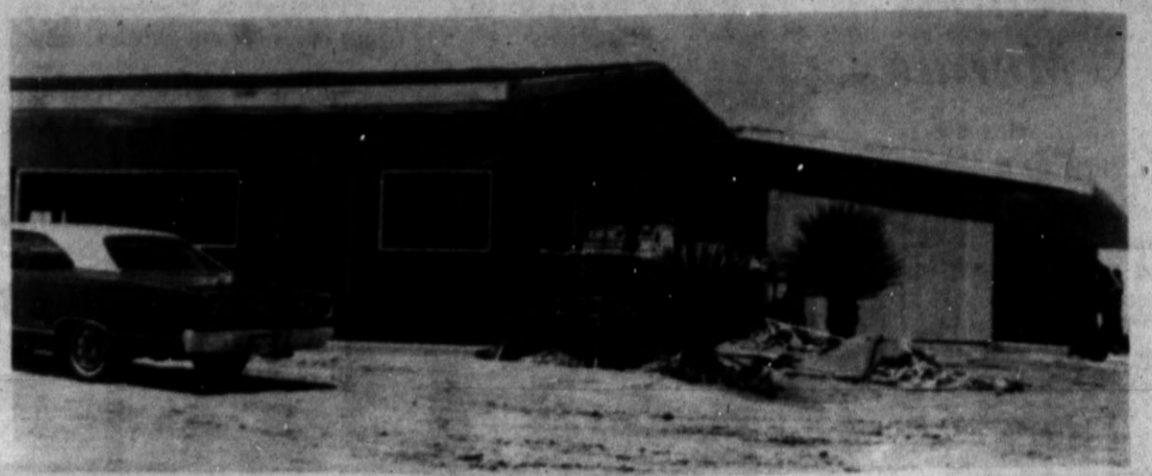
"ROADRUNNER" IN ACTION — The Roadrunner truck stop, located on the old Benefield corner of U.S. 60, is in the rapid process of construction. Owned by Bill Gentry, J. W. Robinson Jr., and Ralph Owens, it is set for completion in mid-May. Opening date is to be announced. —Staff Photo
