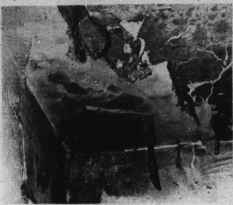
FIRE DAMAGE — A house at 407 E. 4th suffered damage to the wall and ceiling in the kitchen Saturday afternoon when a coupling apparently came loose on the stove. All units of the Hereford Volunteer Fire Department answered the call and the fire was quickly extinguished. The house is owned by Alvin Smith.
