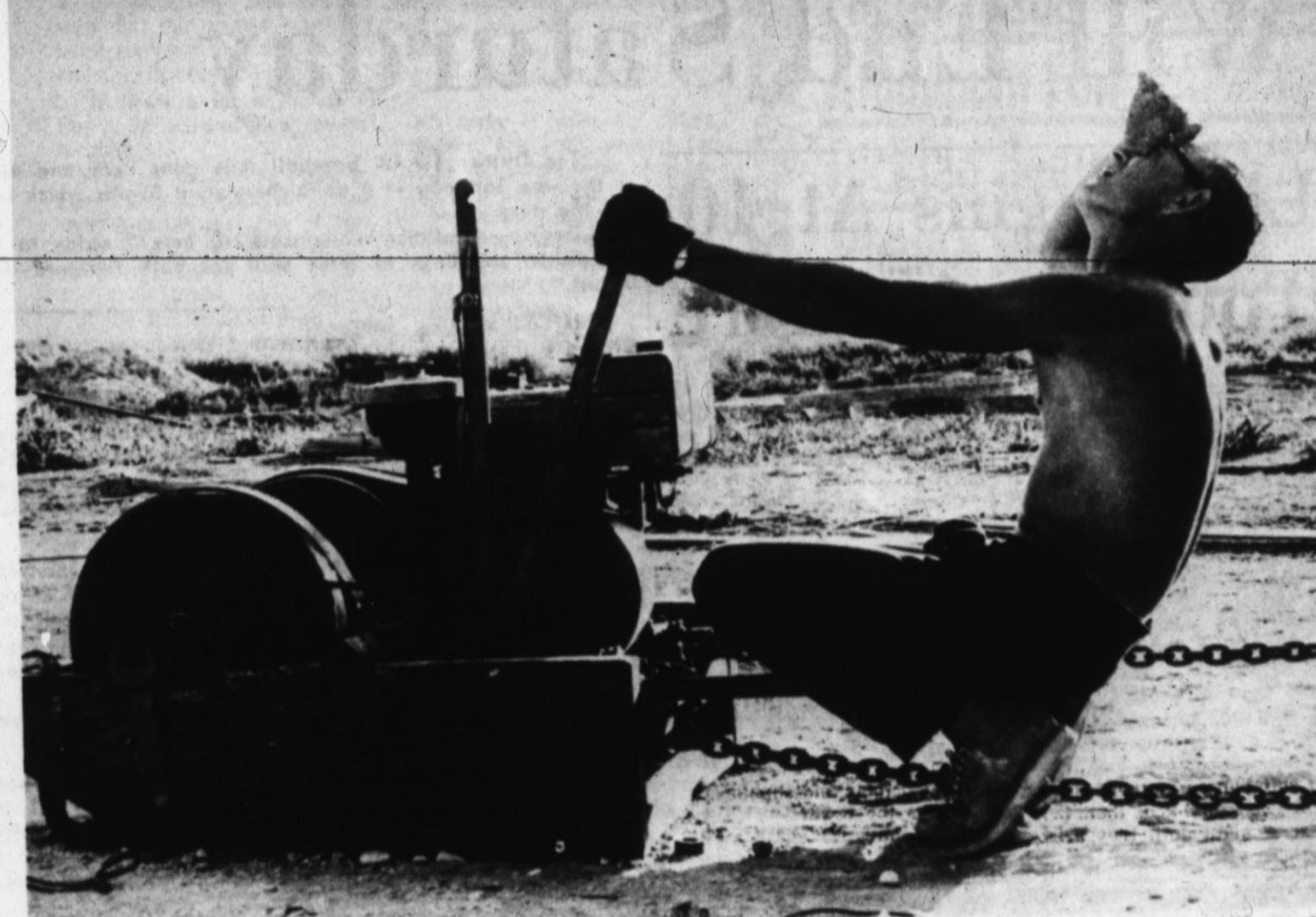
FROM THE GROUND UP — Workmen for the Tri-State Tower Co. of Amarillo start at the bottom and work their way up to the top of their job. That's the way they build towering communications towers, like the one erected here earlier this week. Above, a workman climbs 280 feet above the ground as the 300-foot tower nears completion. Note the bow caused by a stiff breeze against the inch-thick rope used to guide a winch line which runs up through the tower and back down the outside to hoist materials. Workmen say they're "used to" working at such heights amid heavy winds. In the bottom picture, J. M. Duncan operates a small winch — the only mechanization needed by the workmen to erect the skyscraping tower. See story on page 1. (Staff Photos)
