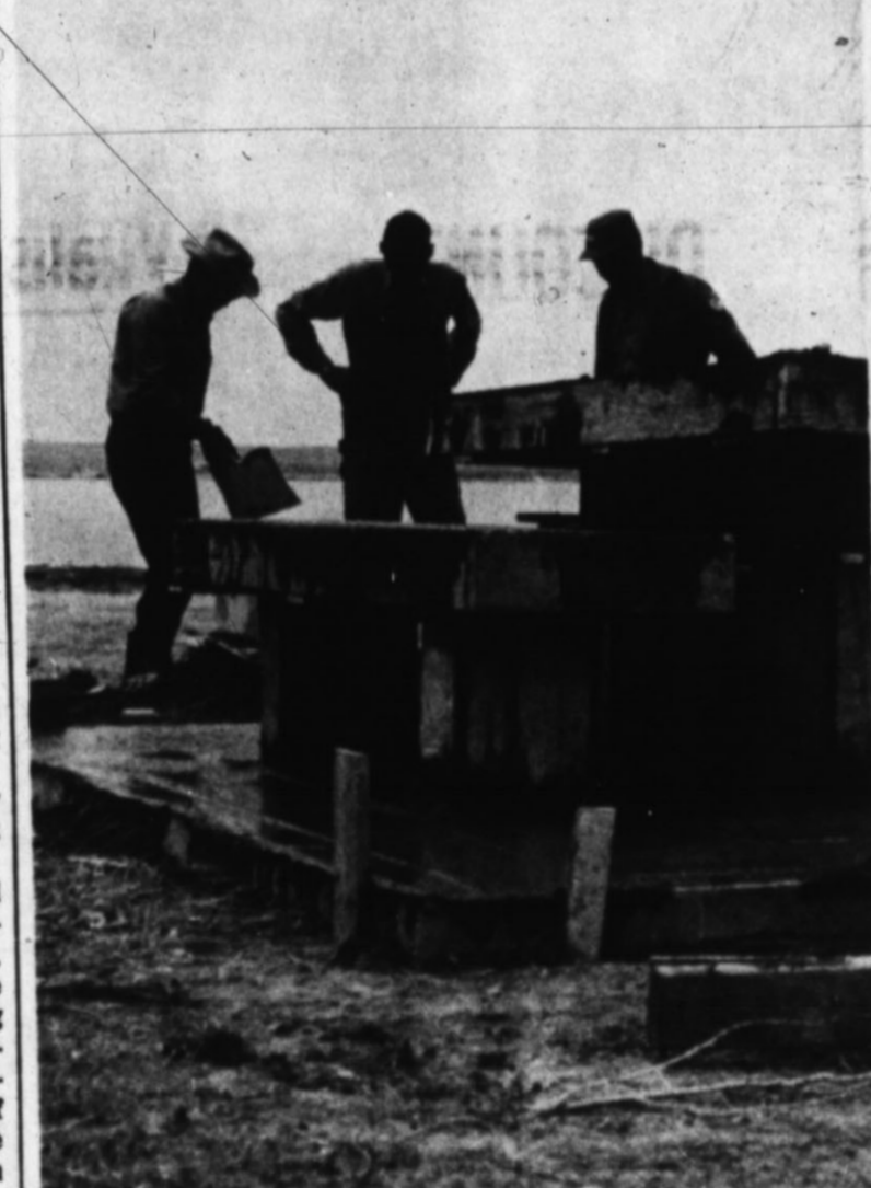
PICNIC FACILITIES — Workmen add the finishing touches to a concrete picnic stand, one of five being prepared for the summer crush at Buffalo Lake. The high usage requires all facilities to be of the strongest design that is economical, says wildlife refuge manager Bob Brown. (Staff Photo)
