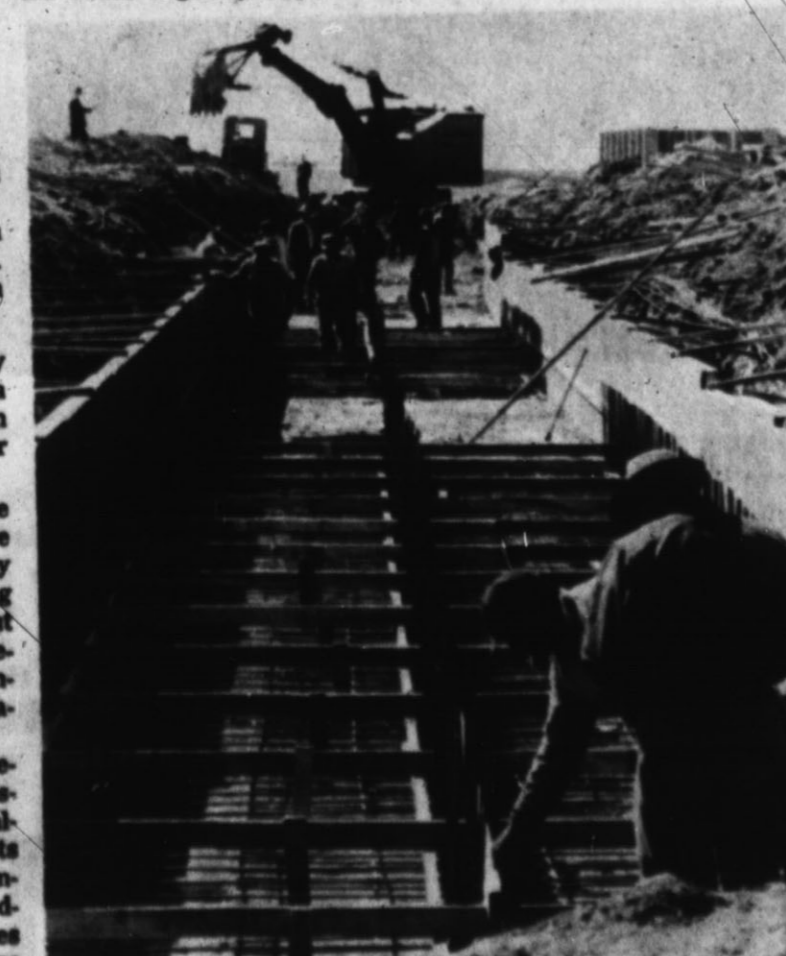
CONCRETE FORMS PLACED — Amarillo construction firm employs follow power scoop Tuesday placing forms for a large storm sewer on Harrison Highway. (Staff Photo)
