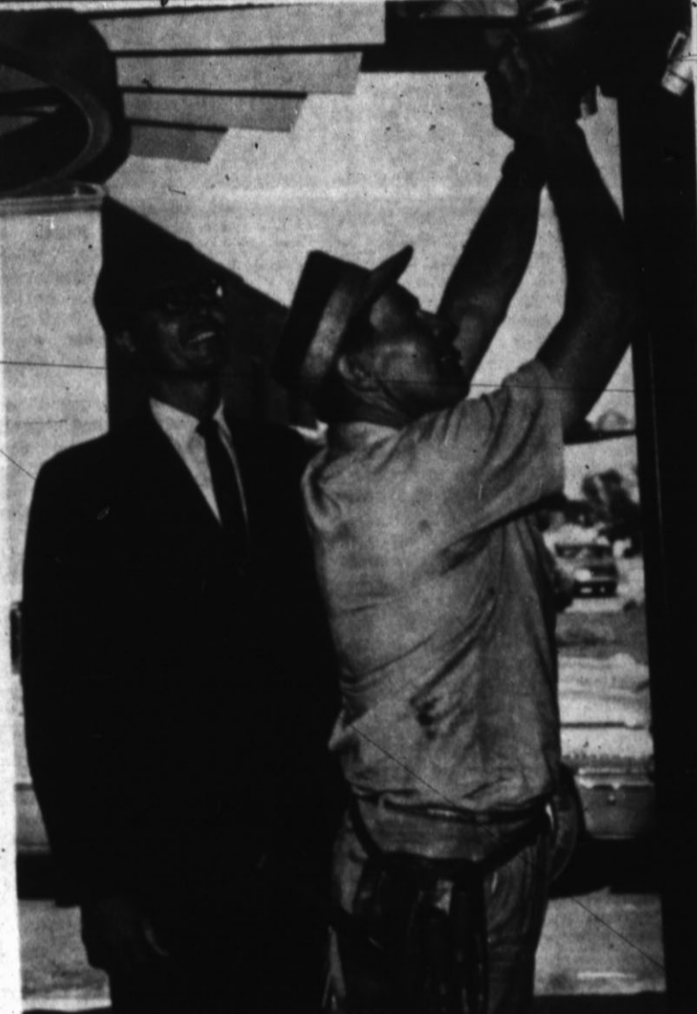
FINAL ADJUSTMENTS — Electrical work on traffic signals and adjustments on lights under the awnings was completed early last week. Charles Owens, local electrician, is shown completing an installation as Melvin Jayroe of Southwestern Public Service discusses the project which will be featured today in grand opening activities. (Staff Photo)
