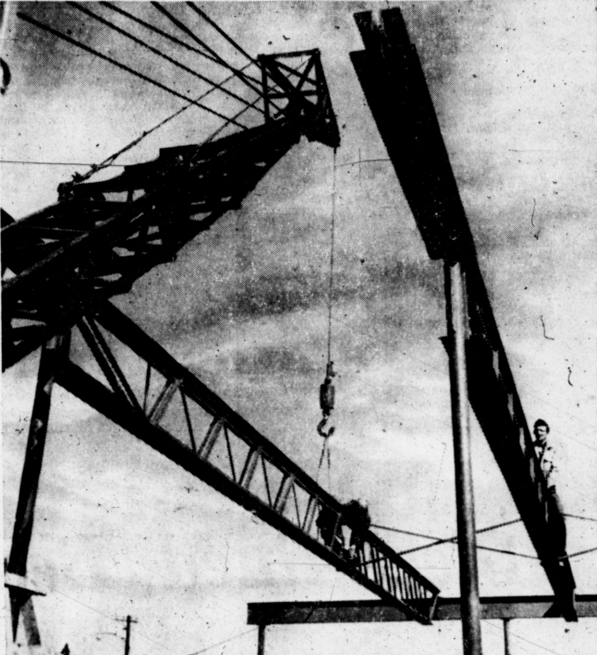
HIGH STEEL for higher education . . . Riggers this week have been putting up steel beams which will support the roof of the new cafeteria and administration quarters in Hereford. The building will be located just south of the high school and will be used by both junior and senior high students. There will be offices for all school district officials and administrators. (Staff Photo)
