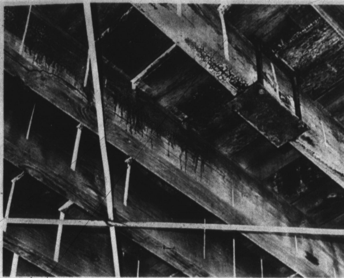
ROTTING AWAY — Timbers supporting this bridge located 1 mile west and 3 1/2 miles south of Dawn show the effect of "too many years" as they begin cracking and rotting away. (See story, Page 1.) The steel saddle (upper right) along with several others, have been placed on the timbers for additional support. (Brand Staff Photo)
