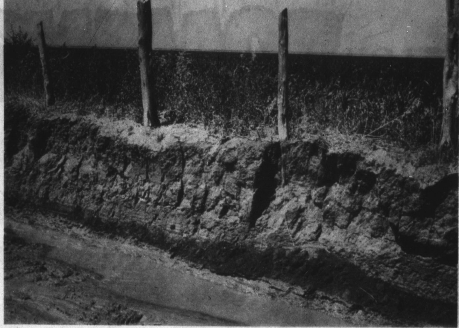
ERODING FENCE LINE — The above photo shows where tail-water has eroded the west bank of a ditch 19 miles west of Hereford. The tail-water is the center of a disagreement between neighbors north and west of the Westway community. (Brand Staff Photo)
