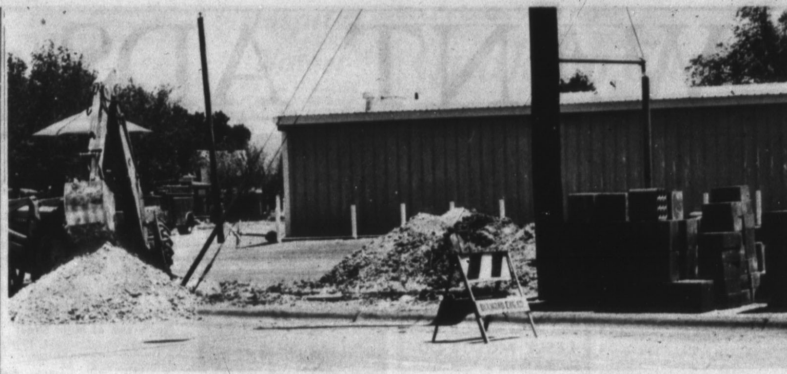
GOING UNDERGROUND — Telephone connections for the northwestern part of Hereford are being laid underground this week. The work has been taking place on Miles Avenue and Park Avenue. This scene is on Park Ave. (Brand Staff Photo)
