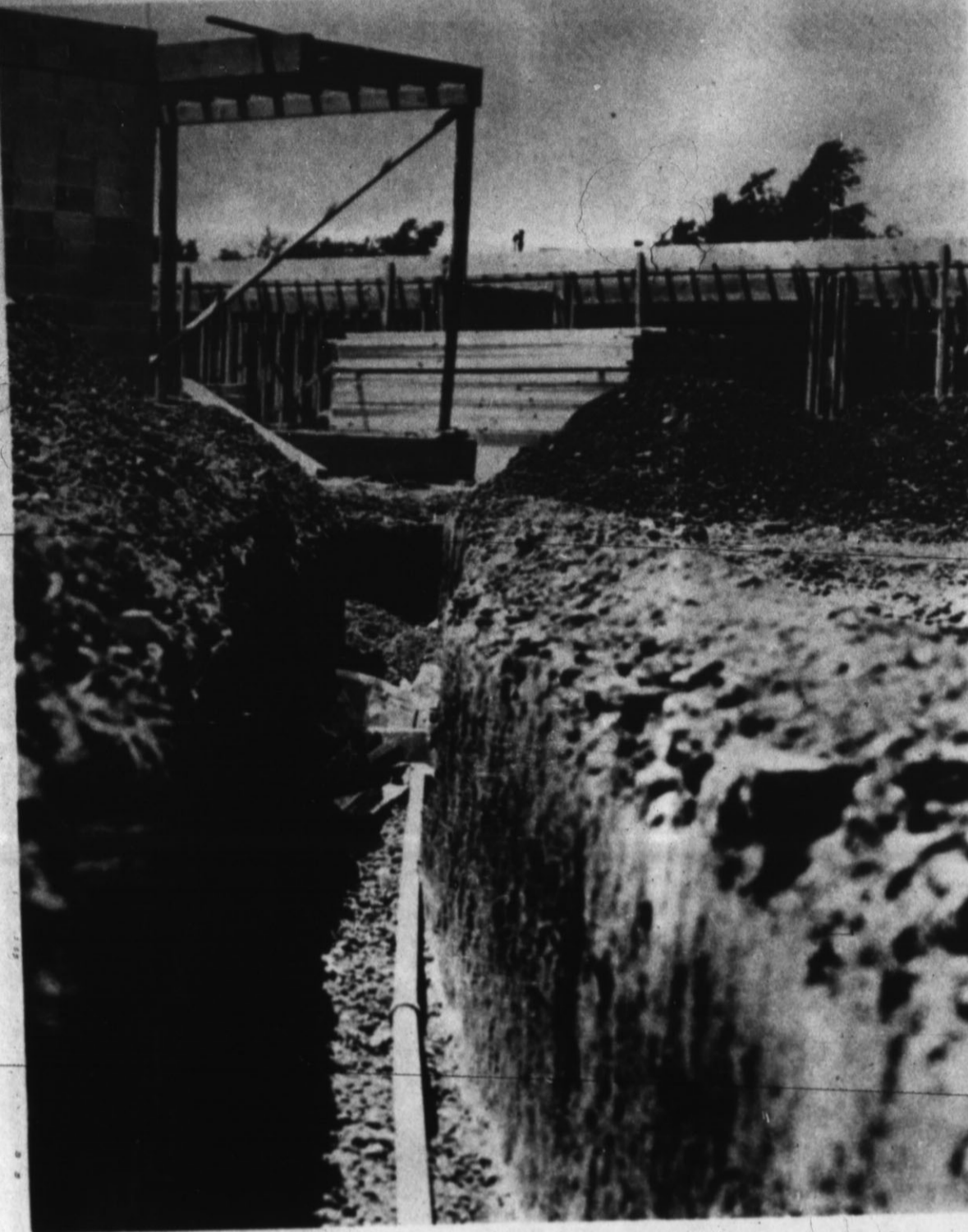
FROM THE GROUND UP — This quarter-million dollar motel is being constructed near the intersection of U.S. Hwys. 385 and 60. The complex will also include a restaurant. It's one of several construction projects now underway in Hereford. (Staff Photo)
