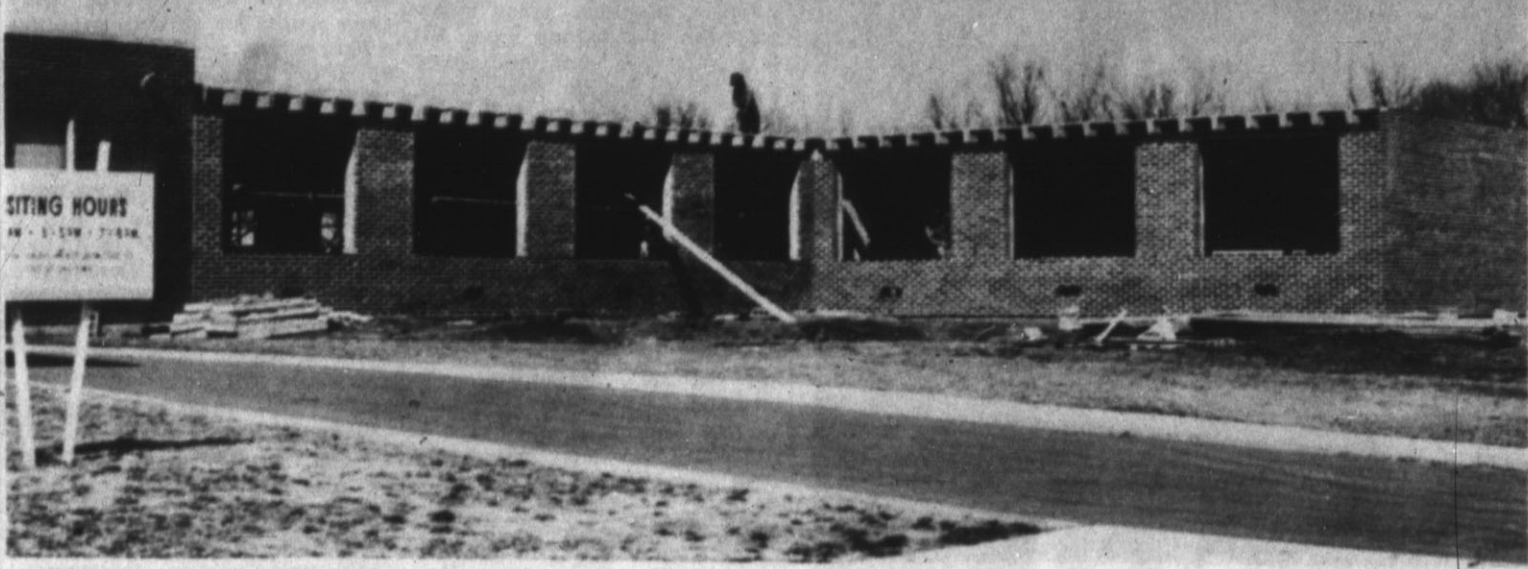
HOSPITAL MAKES PROGRESS — Deaf Smith county Hospital's expansion program is making progress, county commissioners were told at their meeting here Monday, and work is going ahead on schedule. Here's a close-up of the annex. (Brand Staff Photo)
