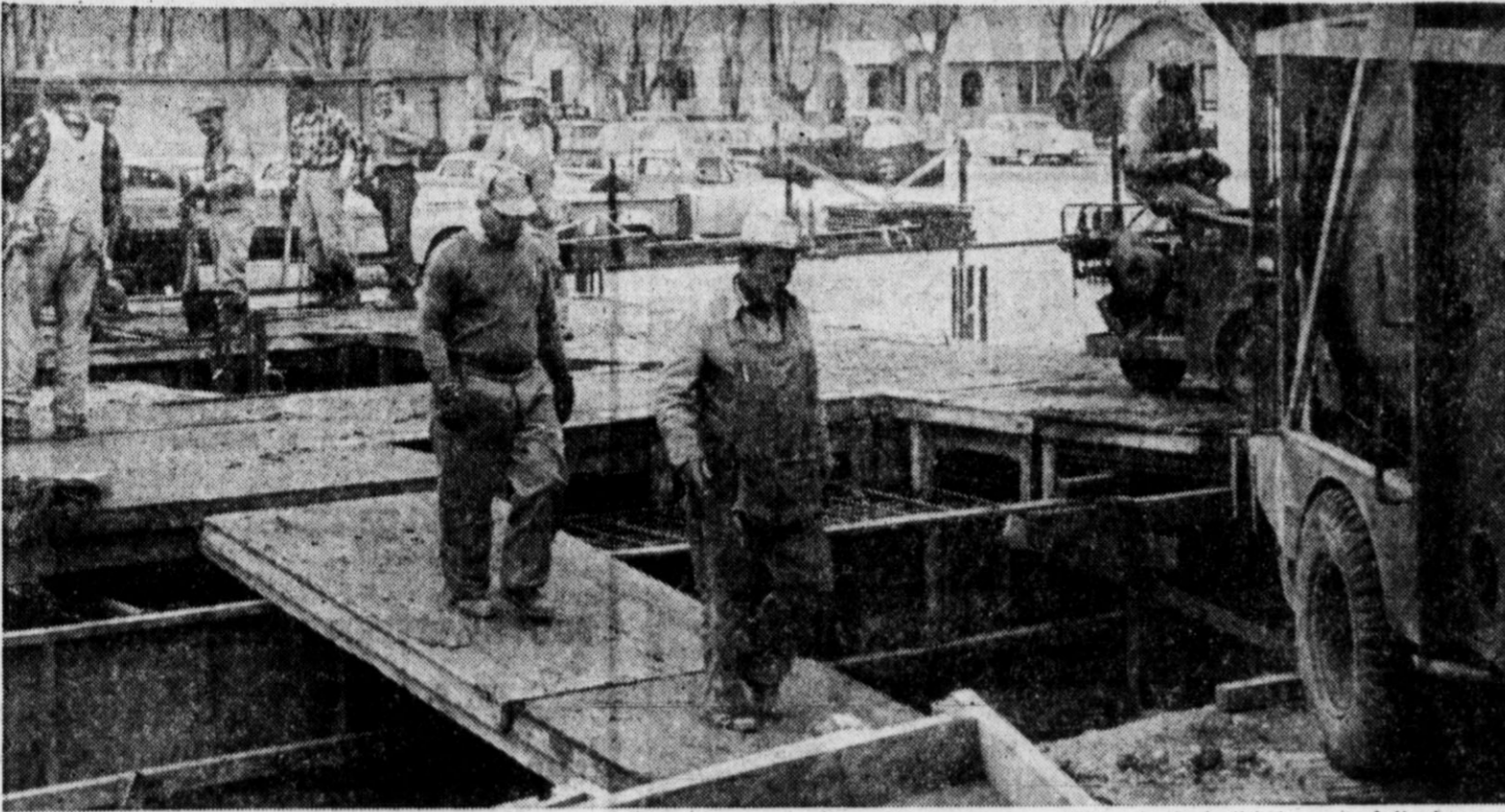
NOW, GOING UP—Work on the new "Emerson 4" building, Southwestern Bell Telephone Company's cross-bar dialing exchange to serve the Hereford area, will be more apparent to onlookers from now on. For several months, work has been confined to digging the basement and foundation for the structure, but this week the first floor was poured over heavy steel reinforcements and forms were ready for the next step upward. The building, at Fourth and Miles, will have about 1,100 cubic yards of concrete in its two
