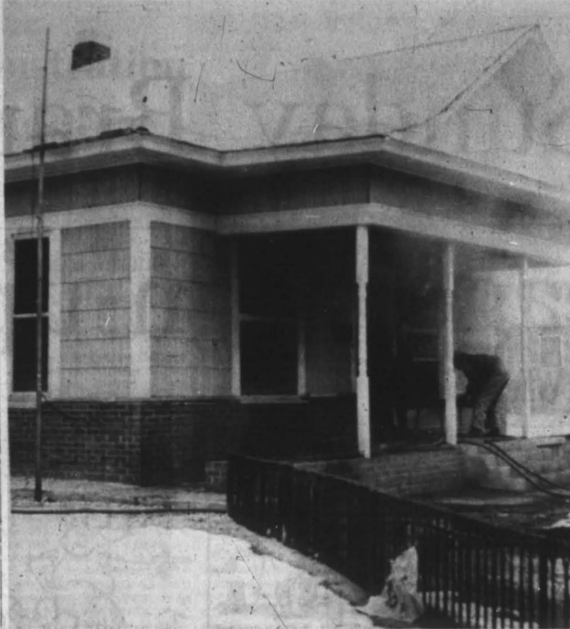
RESIDENCE DAMAGED — Firemen battled a blaze at a residence at 607 N. Main Friday morning which left extensive damage to the R. J. Collier home. Interior of the house was damaged heavily, especially the living room. Loss is expected to run around $10,000. (Brand Staff Photo)
