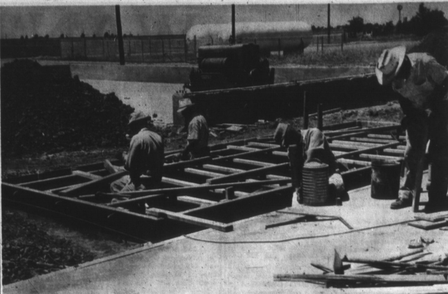
INSTALLING SCALES — Workmen are shown installing scales on the new Shamrock complex now under construction West of Hereford on the Holly road. At completion, the complex will house a complete farm store, plus a service station, offices and butane and fertilizer businesses. (Brand Staff Photo)
