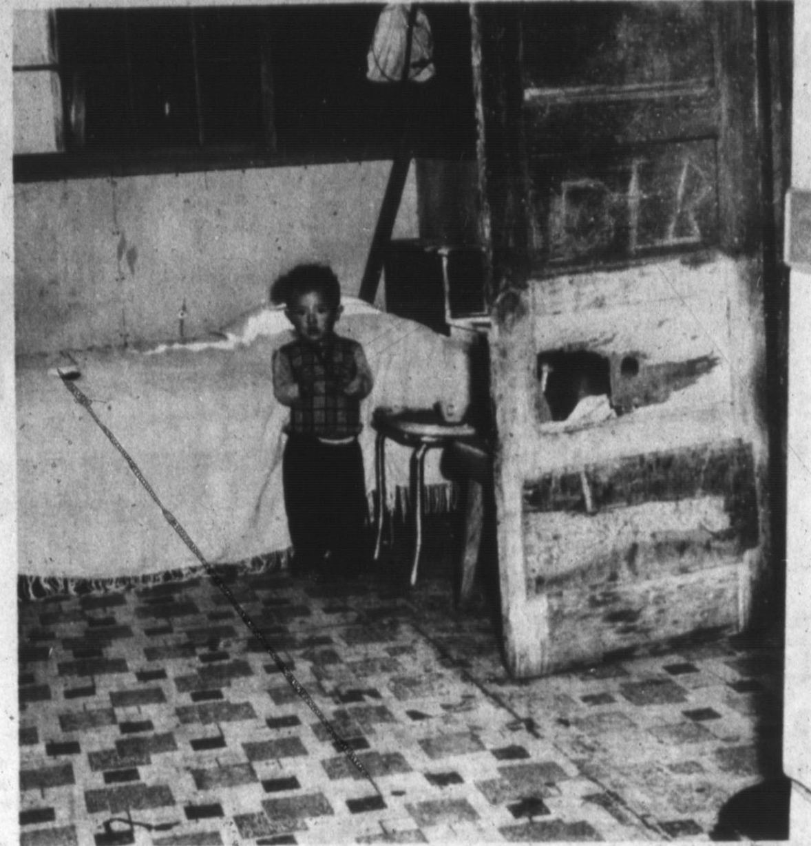
HOLE IN THE DOOR — This shows the condition of the housing in which some of Hereford's migrants live. Note the absence of doorknob, also absence of sheetrock on half of wall. (Brand Staff Photo)
