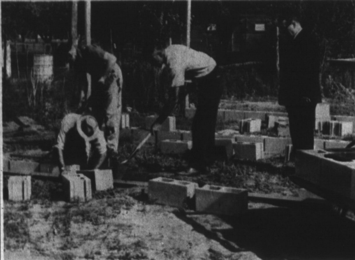
READYING FOR CRUSADE — Volunteers the Latin-American New Life Crusade which Saturday were busily putting finishing touches on the speakers' and choir platform for the Latin-American New Life Crusade which opens tonight. The preaching series will be staged on a vacant lot at 5th and Main. (Brand Staff Photo)
