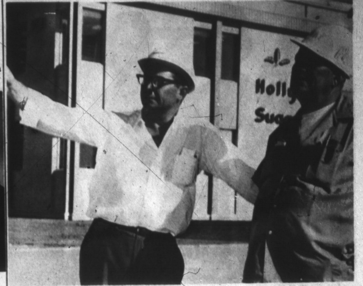
SHOUP PLANT BUILDERS — Bob Harris, will complete the job for Holly Sugar Corporation, shortly after the first of the month. Project Foreman R. D. Wilson, left. The men (Brand Staff Photo)
