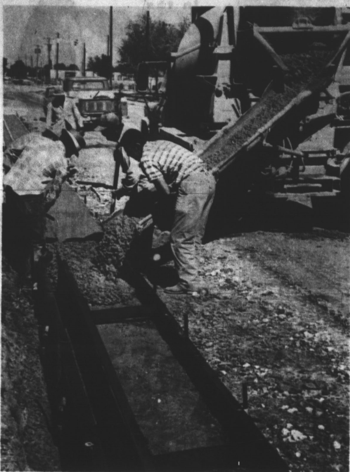
GRAND AVENUE PAVING PROJECT was well underway here this week as workmen were finishing the pouring of curbs and gutters. According to the contractor, Louie Squier, the work will be completed on that part of the project this week and preparation for laying asphalt paving is set to begin. When the project is completed, the 44-foot wide paving will extend from Avenue F to 25 Mile Avenue. (Staff Photo)
