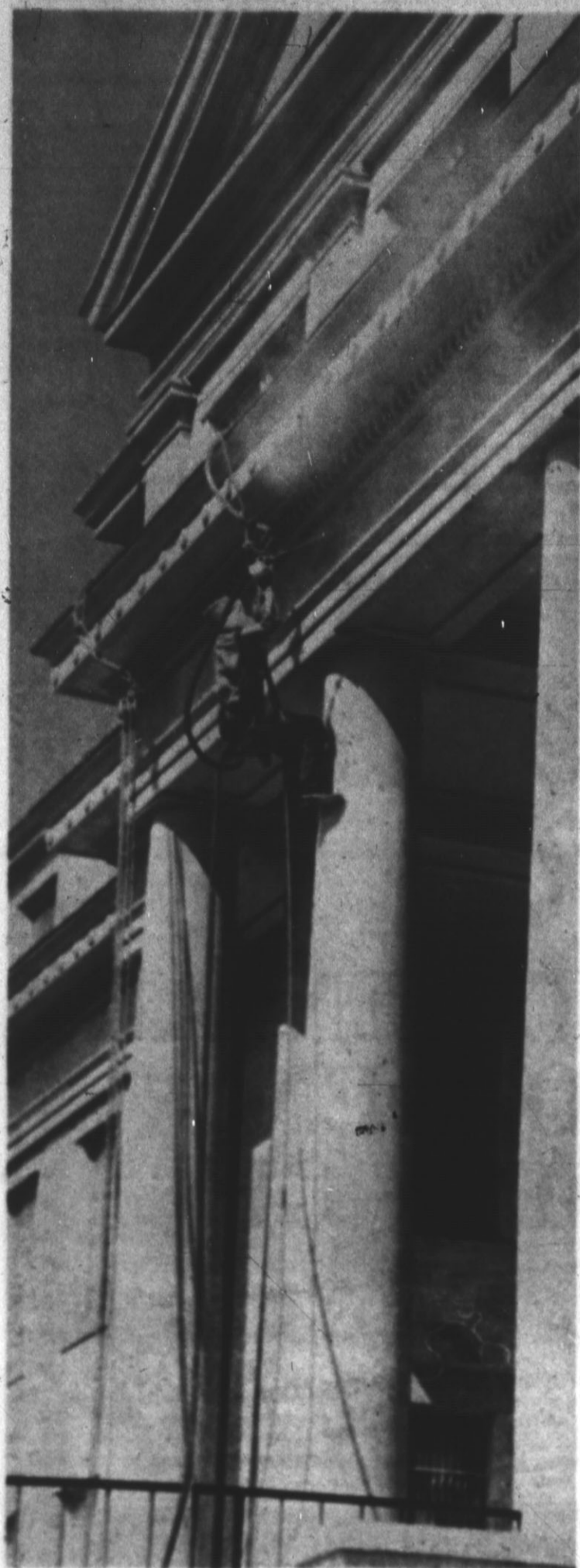
COURTHOUSE CLEANING operations were finished last week and crews began repairing mortar joints in the marble facing of the building. Shown above as he cleans a cement portion of the building, a workman uses a sand-blast unit to remove stains and smooth the surface. (Staff Photo)
