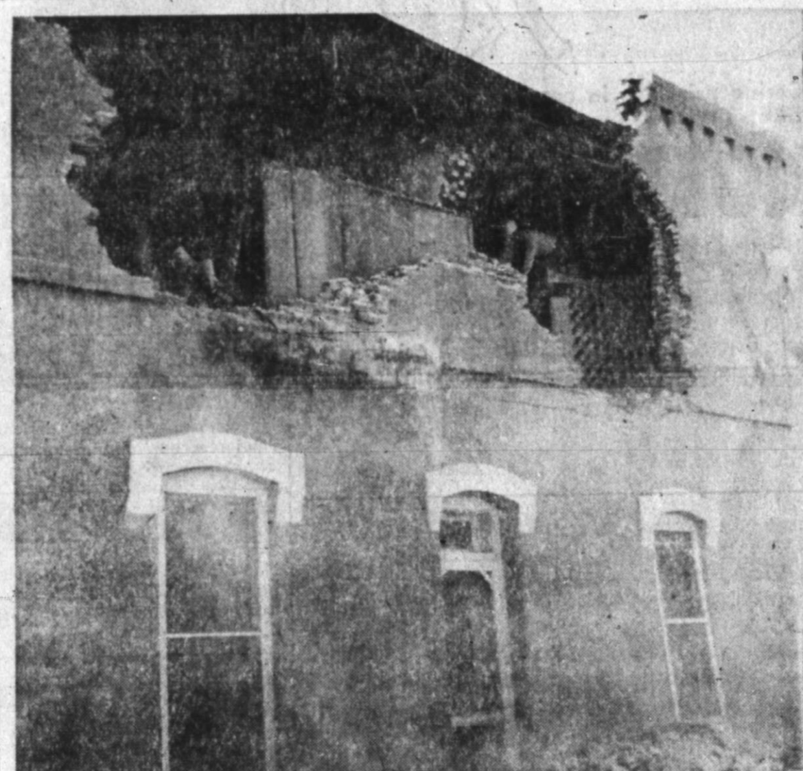
AND THE WALLS came tumbling down, as an Amarillo contractor started razing the old county jail. After removal of much of the roof decking, a winch truck pulled out the imbedded steel window bars. Workers then started prying loose the double brick walls as the landmark began vanishing. (Staff Photo)
