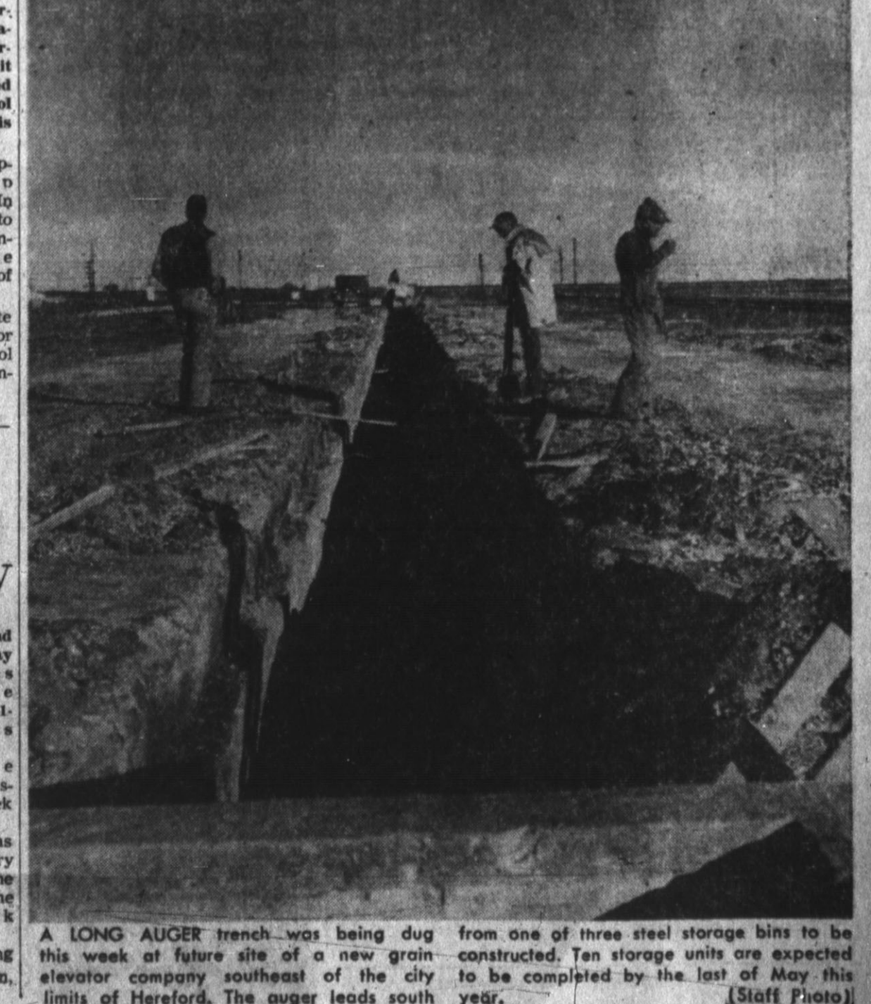
A LONG AUGER trench was being dug from one of three steel storage bins to be constructed. Ten storage units are expected to be completed by the last of May this year. (Staff Photo)
