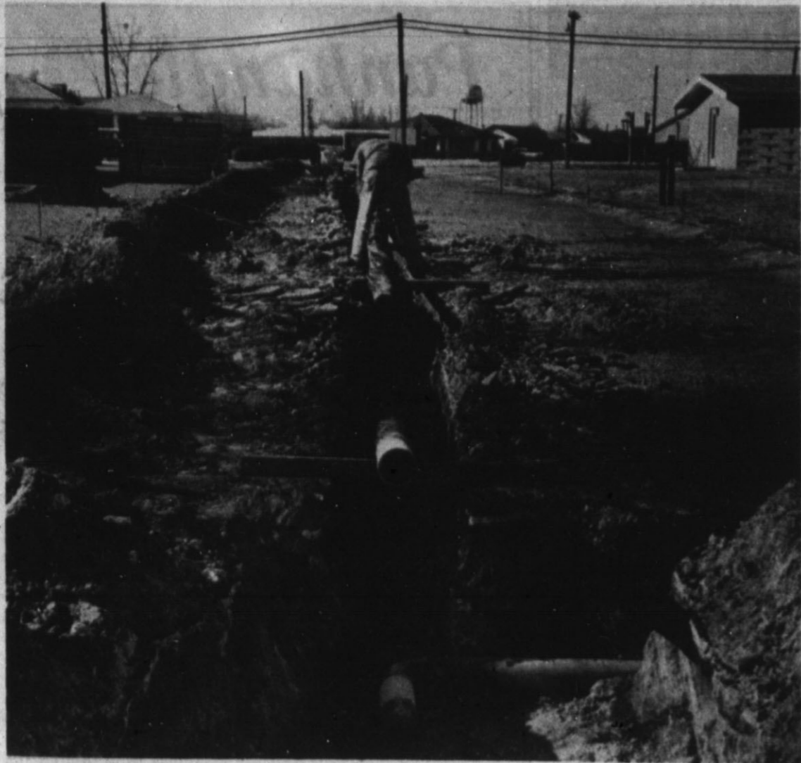
INITIAL WORK STARTED last week on a small addition to the Deaf Smith County Hospital. First order of business was removal of the present gas line and installation of a new line, to avoid having much of the gas under the new building. Construction contractor is Randall Building Company of Amarillo. (Staff Photo)
